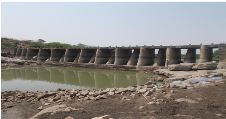
Figure 13 - Few water patch downstream Aihole Barrage
