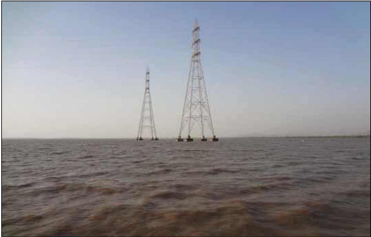
Photo 58: High Tension Line crossing River at Approx. Ch 10.51km
