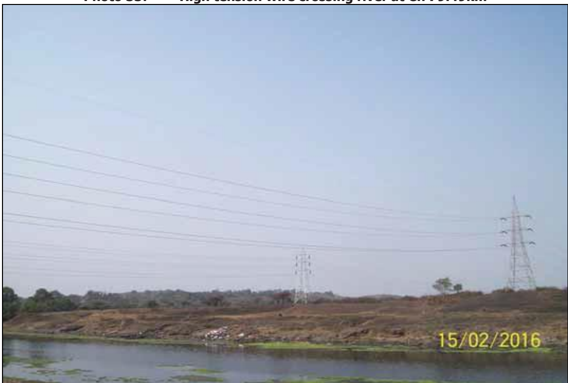
Photo 34: Three sets of high tension wire Crossing River at Ch 81.51km
