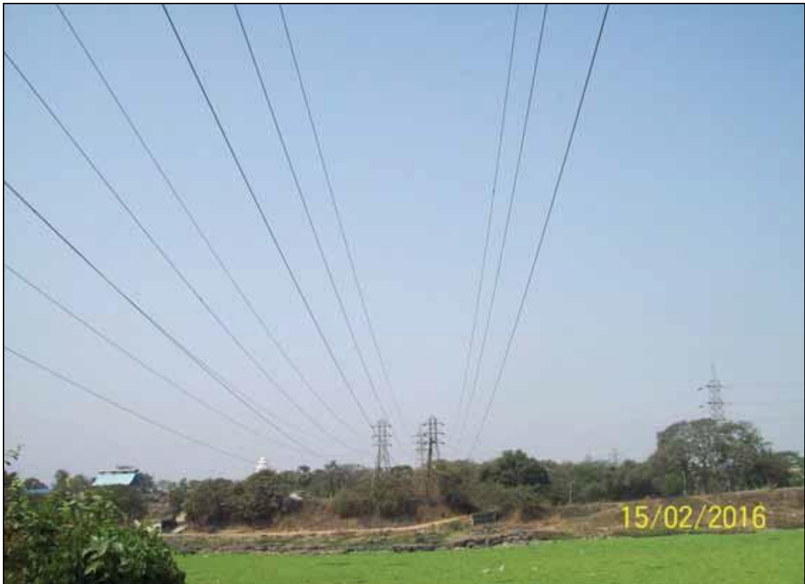
Photo 33: High tension wire crossing river at Ch 79.49km
