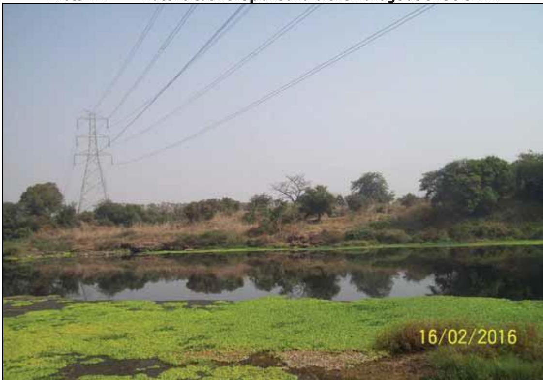
Photo 42: High Tension line crossing river at Ch 100.82km
