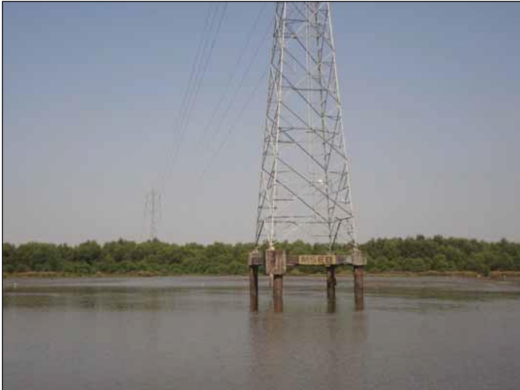
Photo 23: High Tension line at Ch 57.89km
