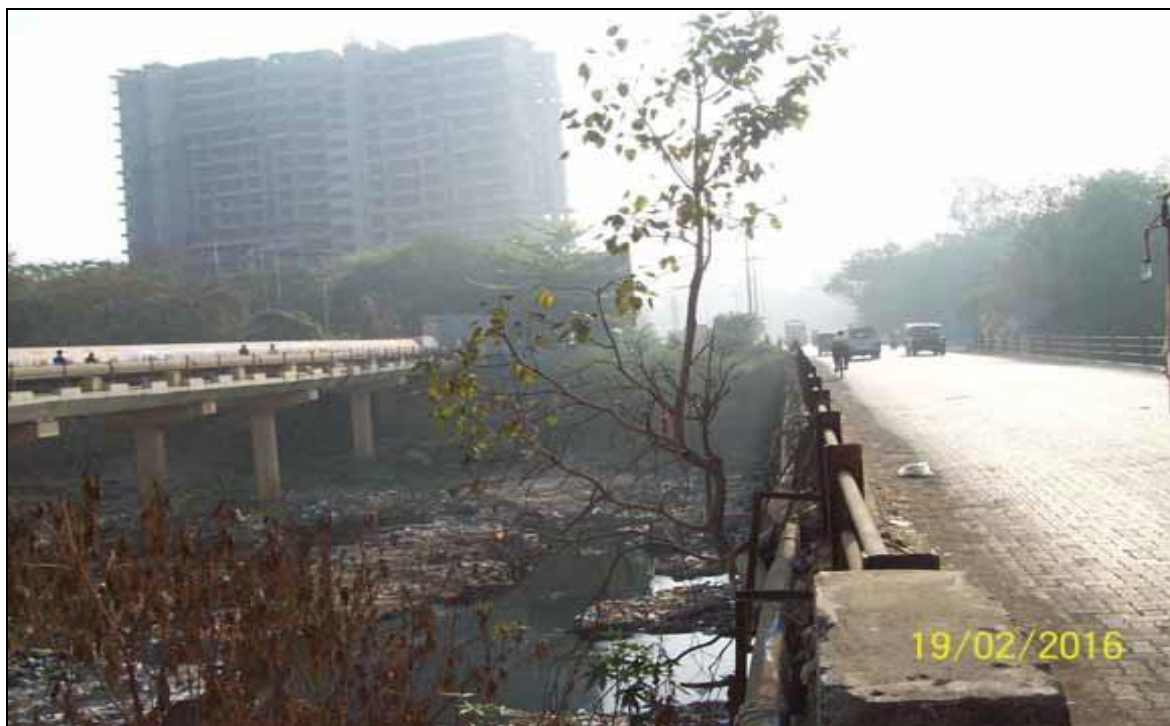
Photo 48: Showing towards east of the Bhiwandi Murwad Road Bridge at Ch 1.33km. Foot over bridge is at 50m north of this bridge
