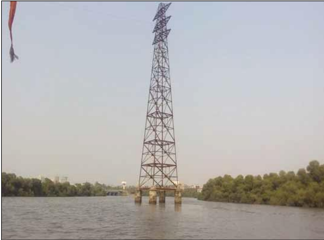
Photo 17: Electric pole in the middle of the river, at Ch 41.43km
