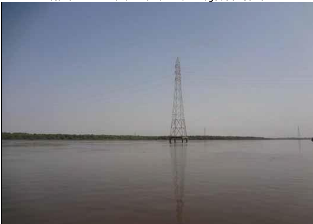
Photo 20: High Tension line at Ch 55.17km
