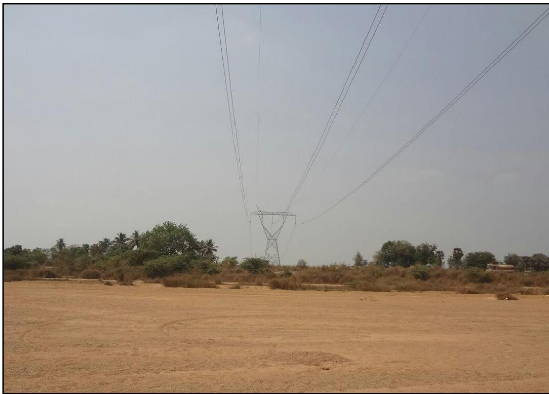
12: HT line at Chainage 28.3
