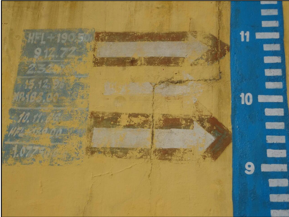
17: HFL on Ellis Dam at Chainage 47.3 km
