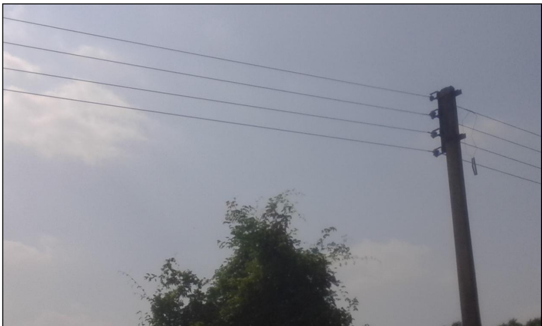
Figure 7- Electric line (Chainage-11.936 km)
