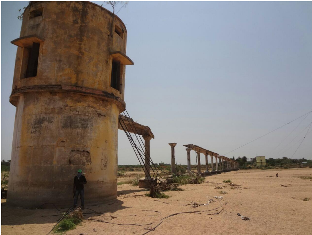
30: Old water Intake from mid of river, VC-7m, HC-8m at ch 117.5 km
