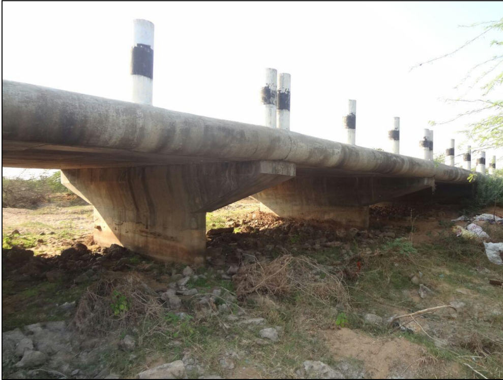
33: Arcot-Kathpali ground bridge, VC -2m, HC -6m, Length -250m at Ch 126.2 km
