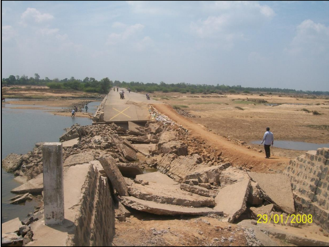
5: Damaged Causeway at Chainage 11.4 km
