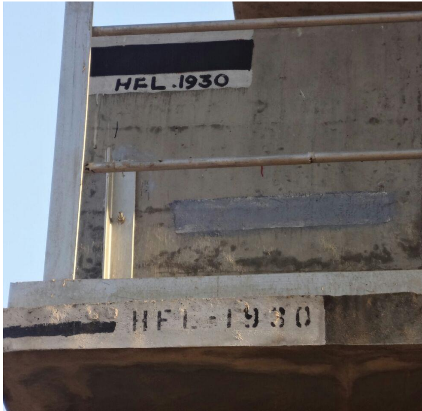
34: HFL mark on pillar of Rail Bridge at Chainage 141 km
