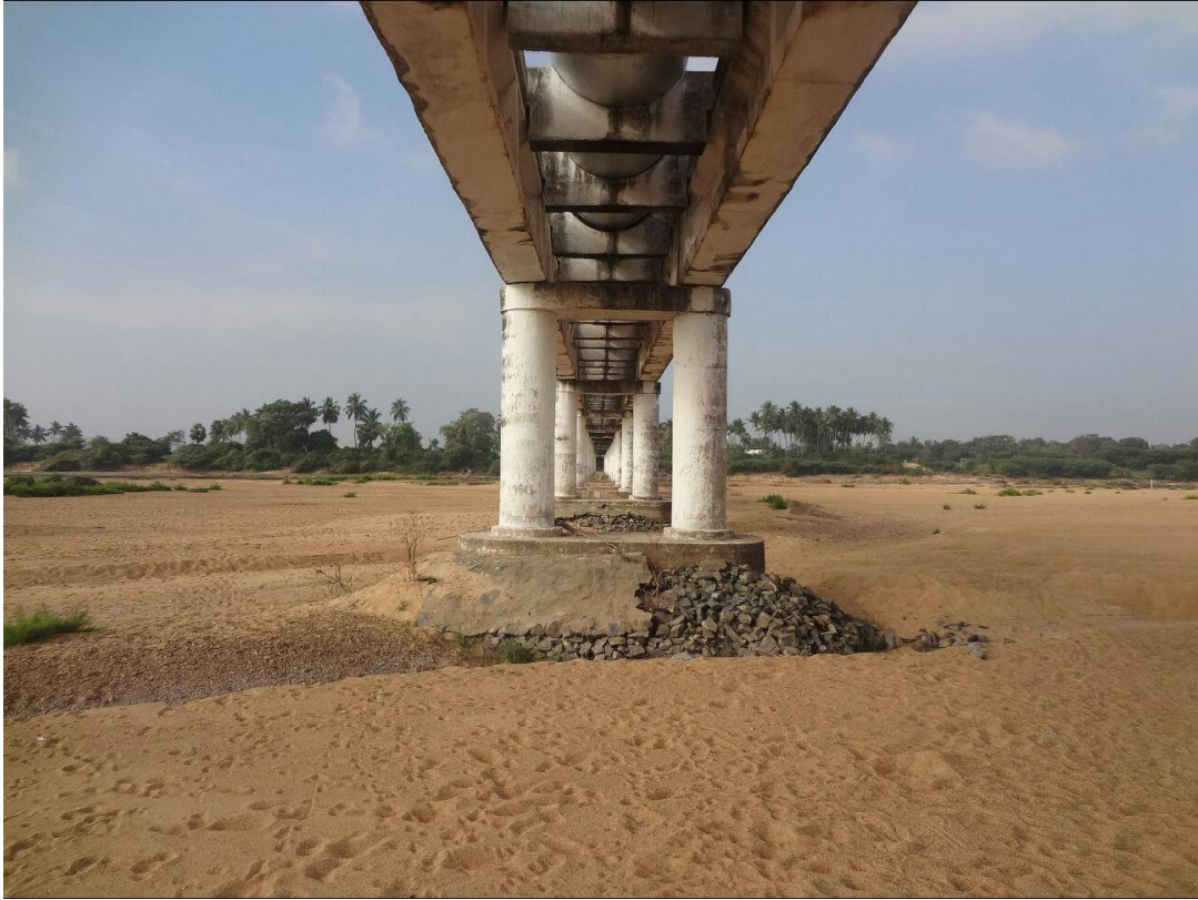
9: water Pipeline Bridge Vertical clearance-6m, HC-17m, Length-800m at ch 18.7 km
