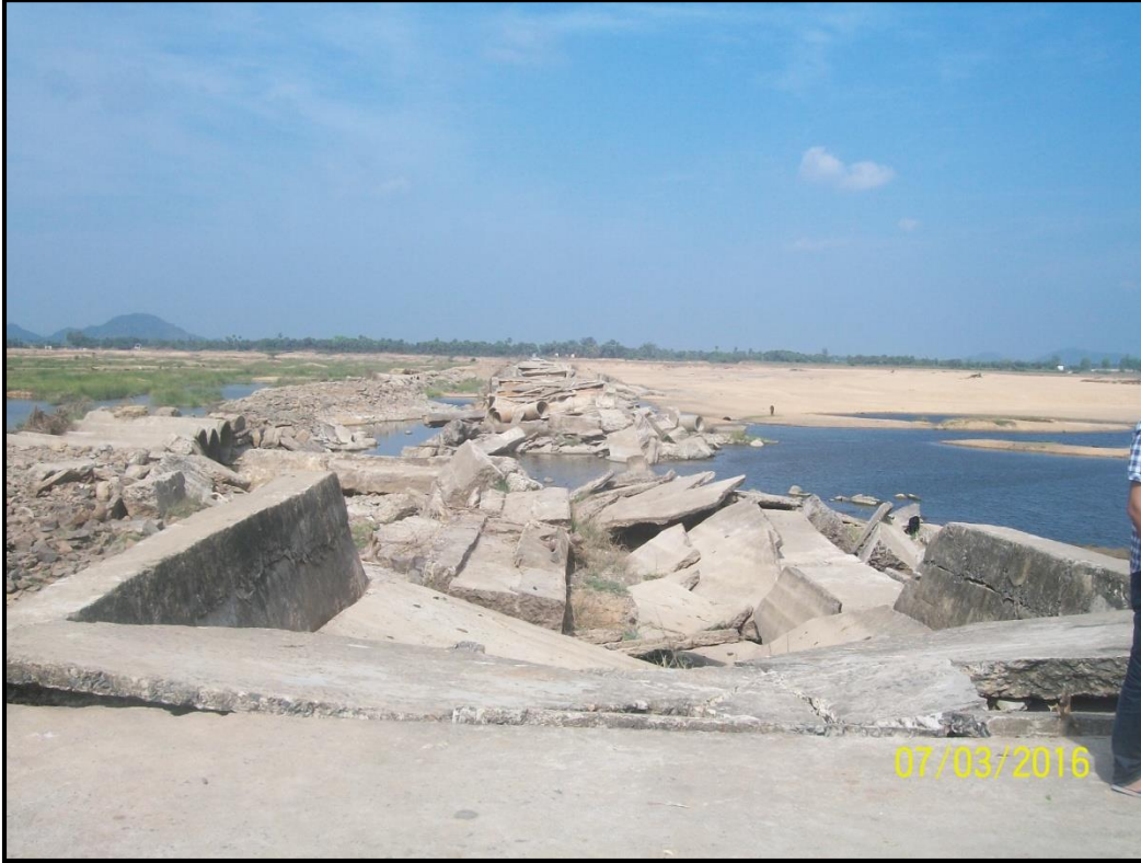
13: PV kalathur road bridge (Damaged Causeway) at chainage 27.3 km
