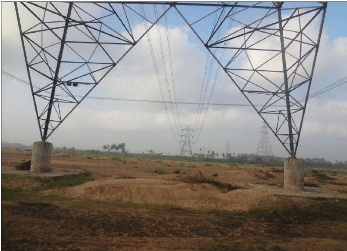
8: High Tension line with HC-400m, VC-15m at Chainage 17.8 km
