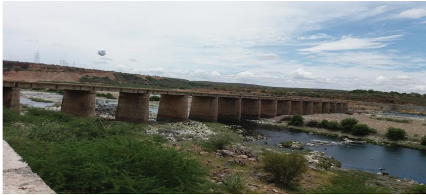
Figure 24 - Broken Bridge at Nagarjuna Sagar (ch. 43.19km)
