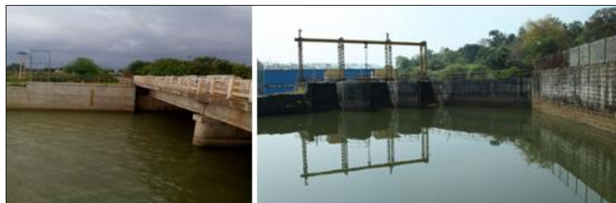
Figure 93 - Small Hydel Power plant at Gugal village (ch. 395.10km)
