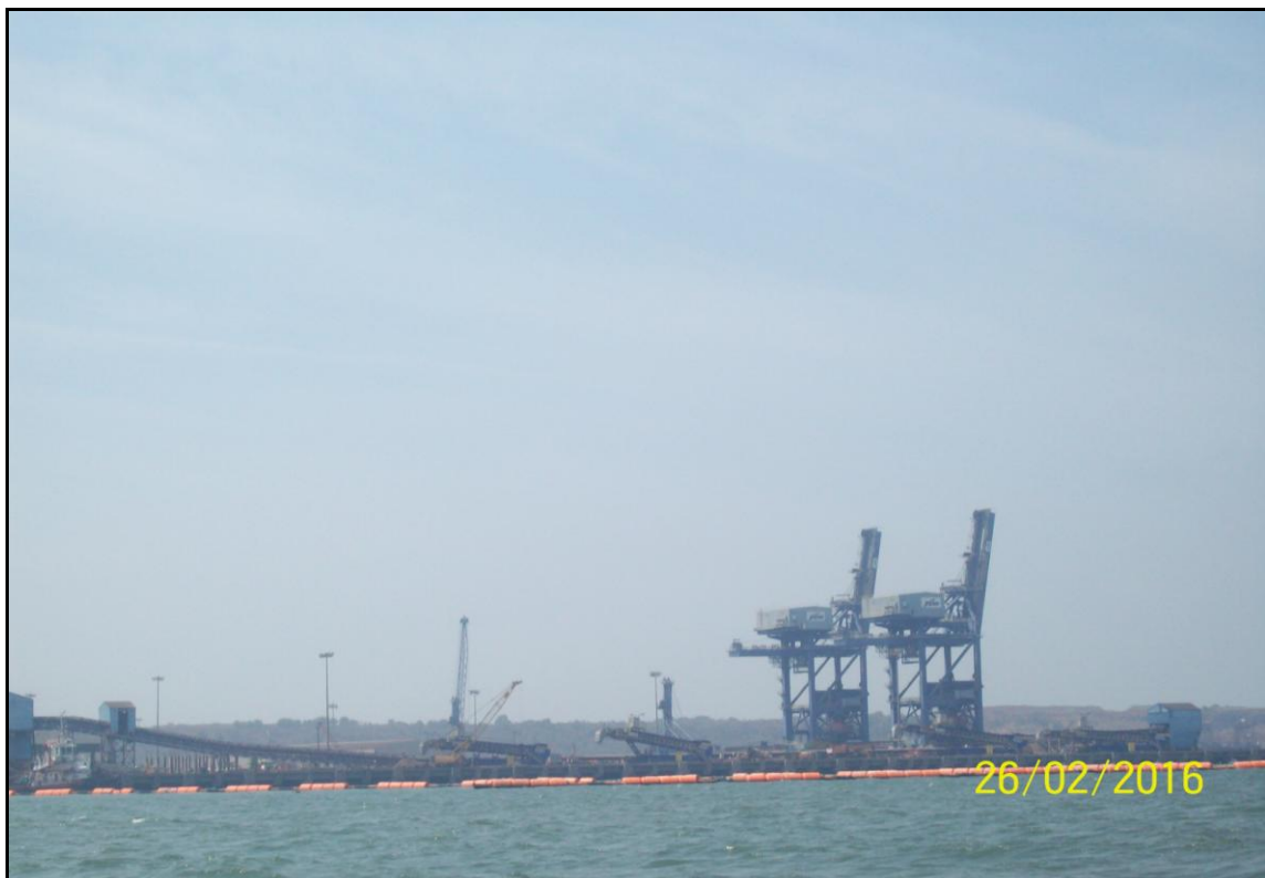
Photo 4: Jindal Port Jetty on South bank. Reclamation work in progress at Ch 1.2km
