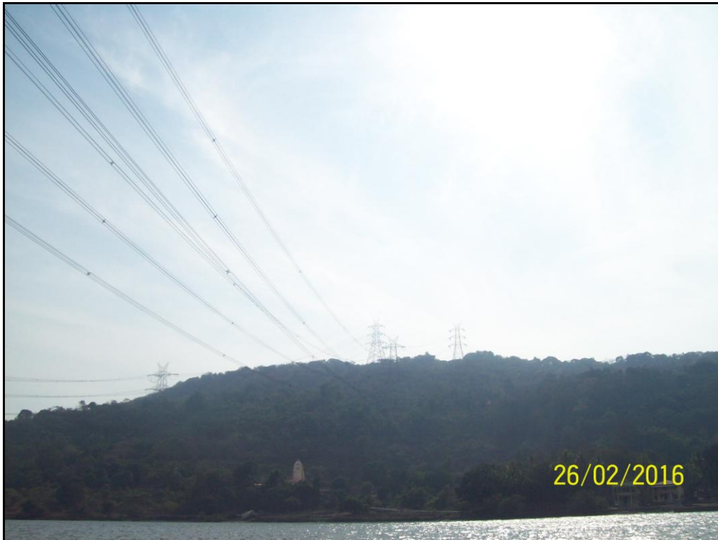
Photo 11: High Tension Line Crossing River at Ch 14.49km (17°16'24.4"N, 73°17'48.8"E)
