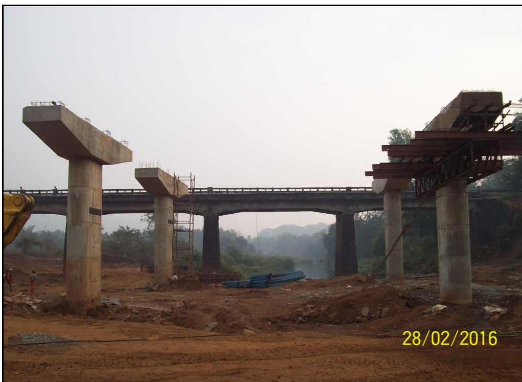
Photo 24: Old Shastri Bridge and Construction of new both way bridge at Ch 53.53km (17°10'01.3"N, 73°32'44.6"E)
