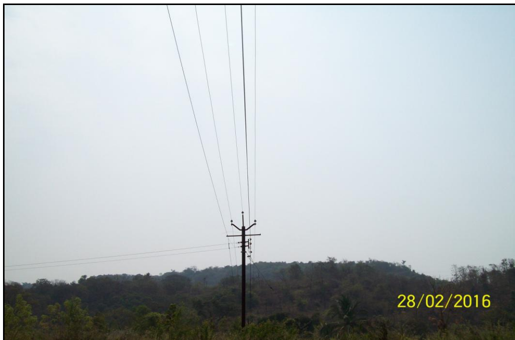
Photo 22: Electric lines crossing the River at Ch 48.98km (17°10'09.1"N, 73°30'36.2"E)
