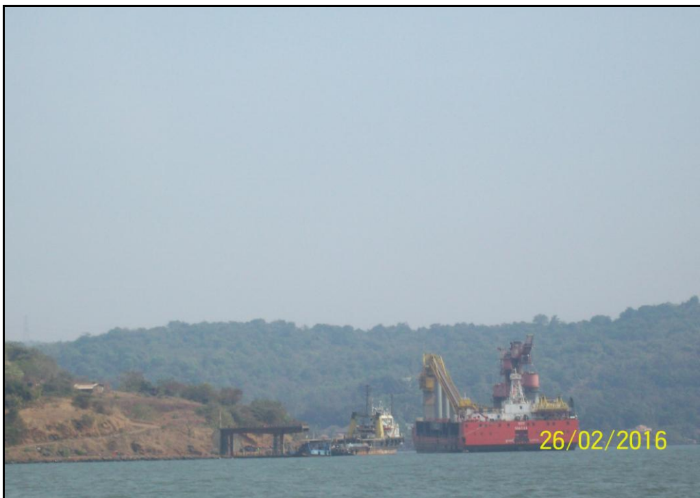
Photo 10: Reclamation on the North bank of river at Ch 9.38km (17°17'33.7"N, 73°16'18.3"E)
