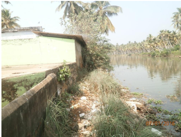
Figure 14-Waste dumping on AVM Canal (1.2 km Chainage)
