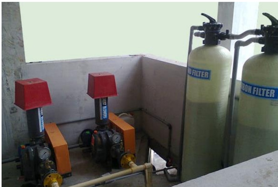
Figure 5.15 Example of a low-cost sewage treatment plant
