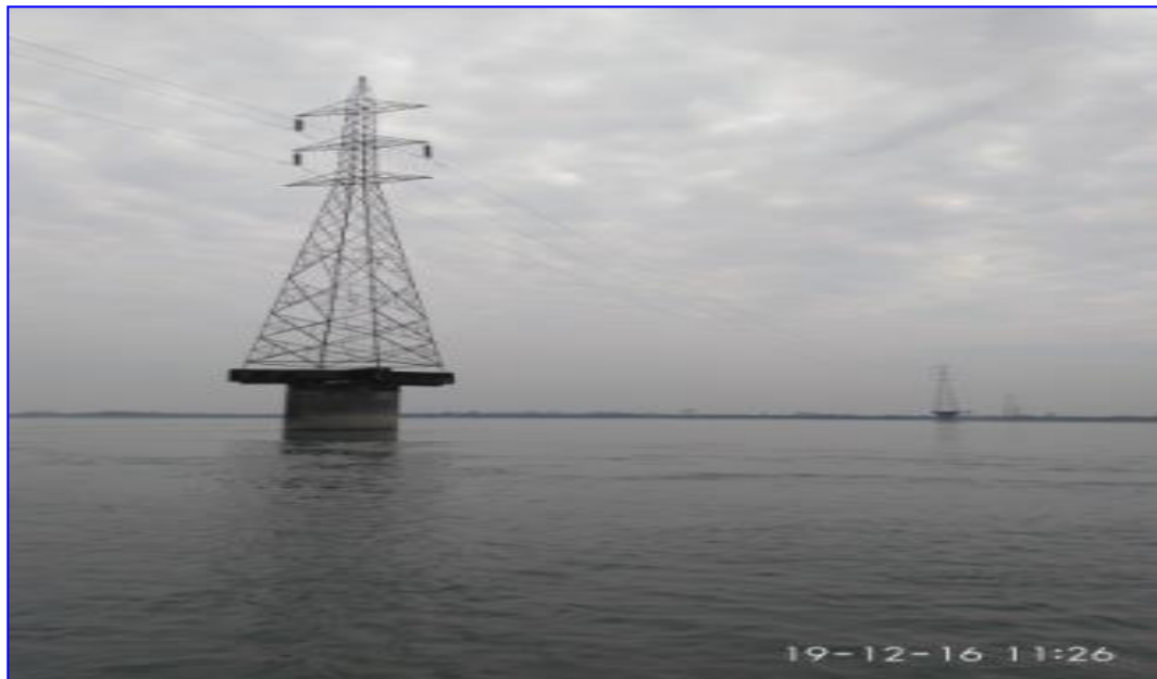
Figure 2.1 High Tension Line at CH 40.4 km – Kabhulighat
