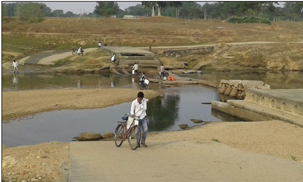
Figure 21- Damage Check Dam (Chainage- 57.949 km)
