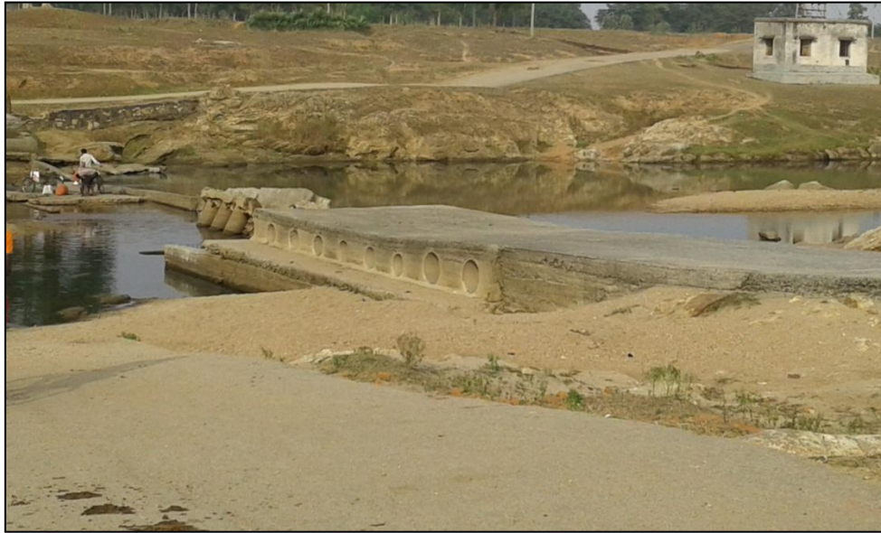
Figure 49-Damage Dam (Chainage- 57.949 km)
