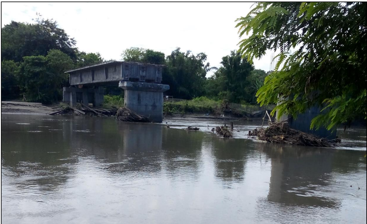
The under- Construction Bridge is situated near at chainage of 34.920km at Satdala Village. The bridge location is (Lat-26°15'24.75"N, Long-91°32'6.95"E).
