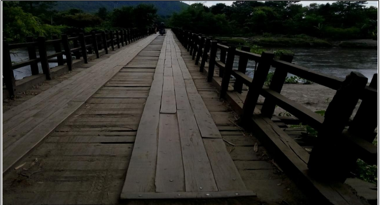
The wooden Bridge is situated near at chainage of 35.348km at Satdala Village. The Bridge location is (Lat-26°15'21.17"N, Long-91°32'22.24"E).
