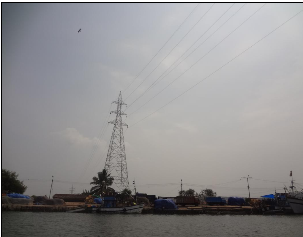
Photo 4: High Tension line Crossing Over River at Ch 2.20km (15°09'33.3089"N, 73°57'12.1275"E)
