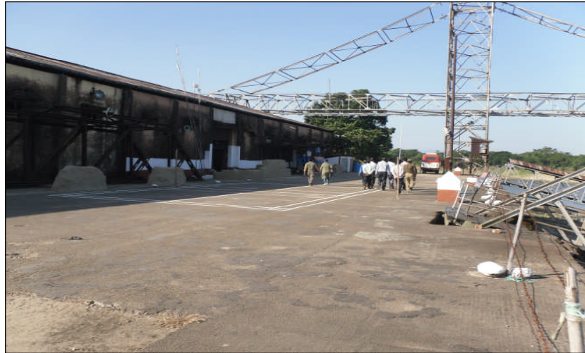
Figure 2.8 View of Cargo Handling Yard & Covered Storage Shed in CIWTC Terminal at Karimganj
