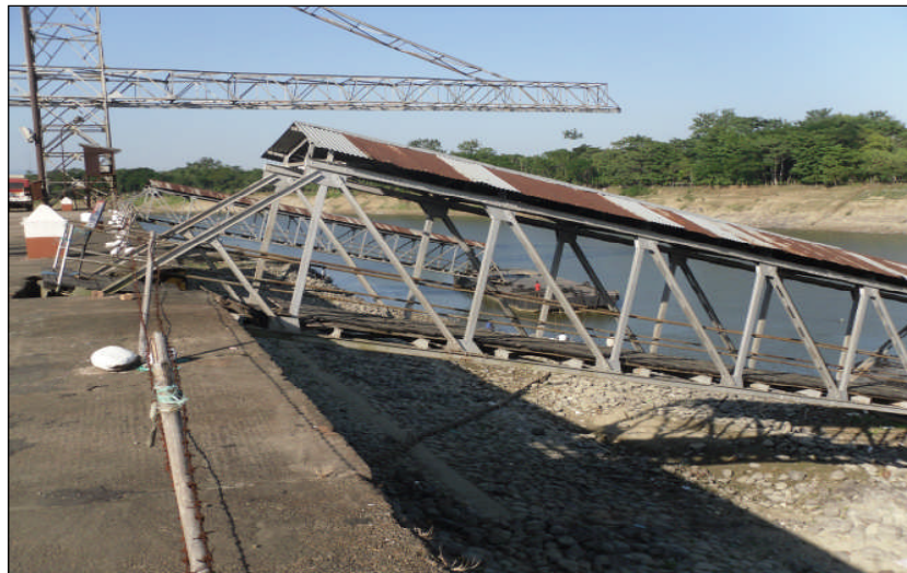
Figure 2.9 View of Gangway with Floating Pontoon arrangement in CIWTC Terminal at Karimganj during lean season flow
