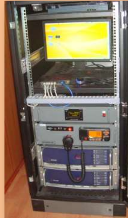
Equipment RIS at Base station
