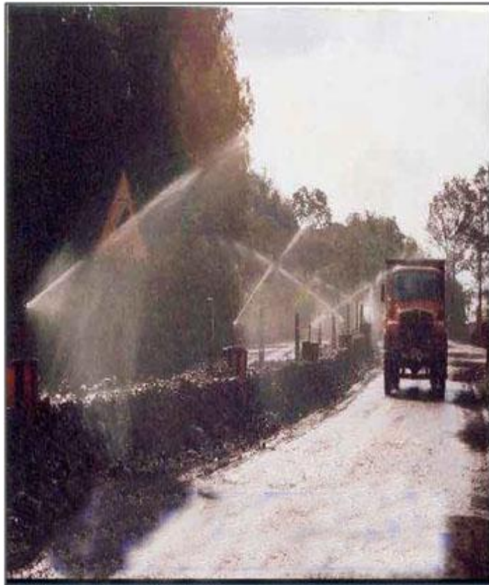
Fig. 5.11: Fixed Water Sprinklers alongside the road as dust suppression measures
