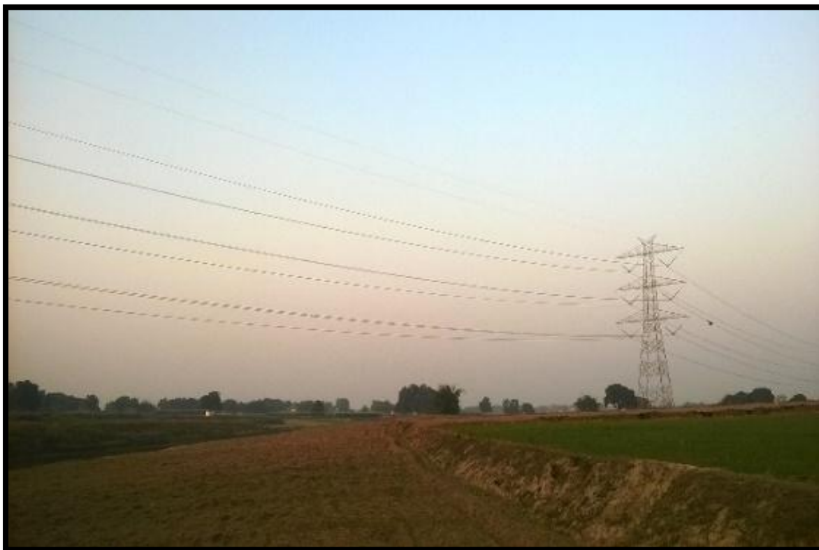
HT Line at Ch 13.25 km
