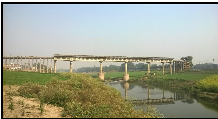
Water Pipe Line Bridge at Ch 2.11 km
