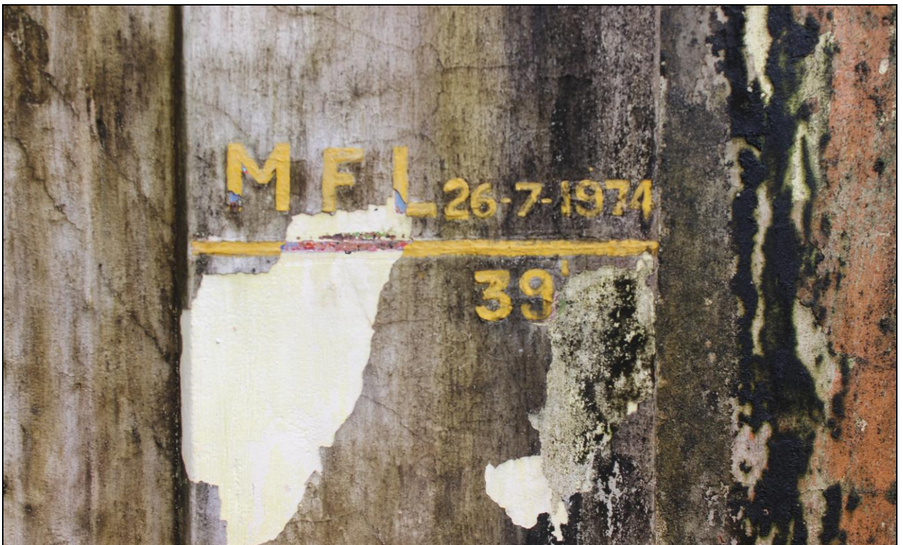
Photo 14: Maximum Flood Level of 39 Ft. Dated 26/07/1974 Mark near Thumbe Barrage at Ch 23.50km
