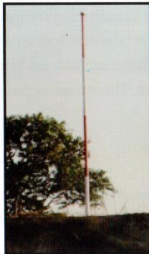
Light on Steel Pole
