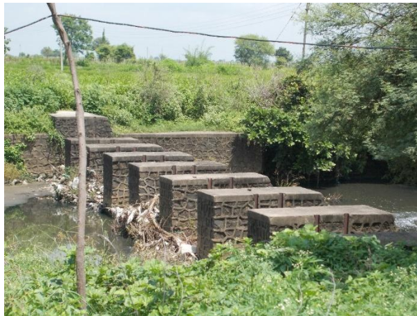
Figure 12 - Damaged Check Dam (33.328 km chainage)
