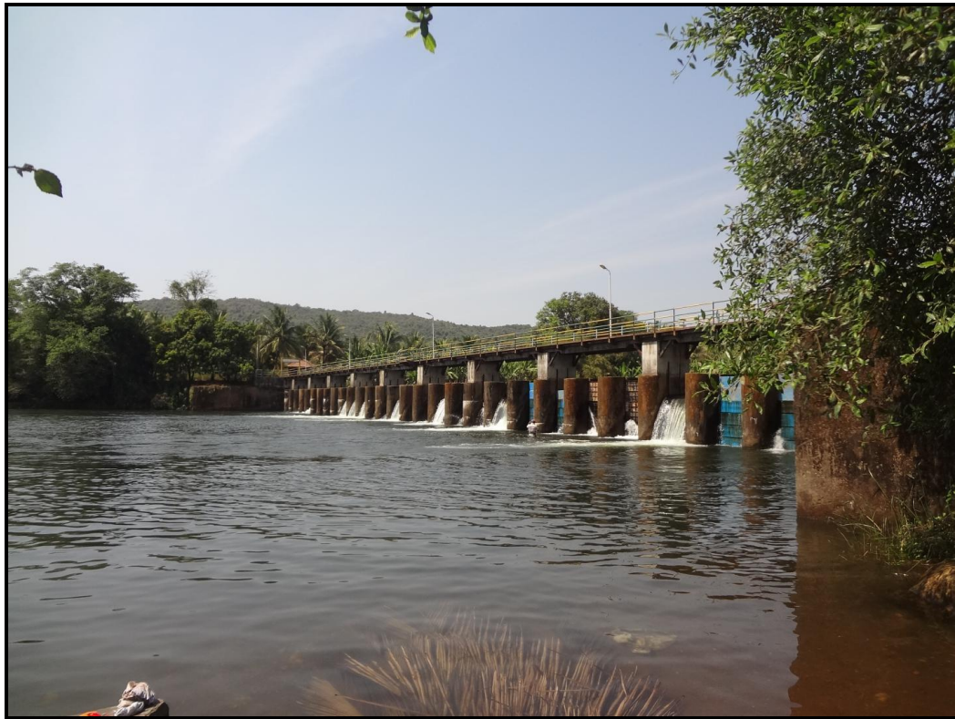
Photo 23: Light Motor Vehicular Bridge over Bandhara, SAL-IBRAMPUR at Ch 28.67km (15° 41' 53.73"N, 73° 55' 42.64"E)
