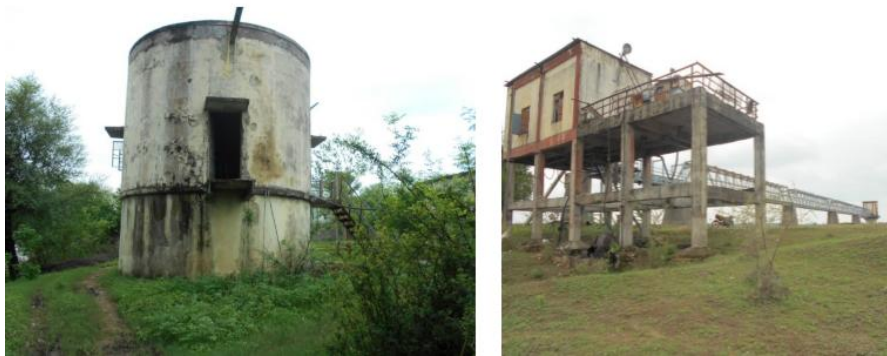
Figure 19 - Pump Houses (129.444 km chainage & 143.828 km chainage)
