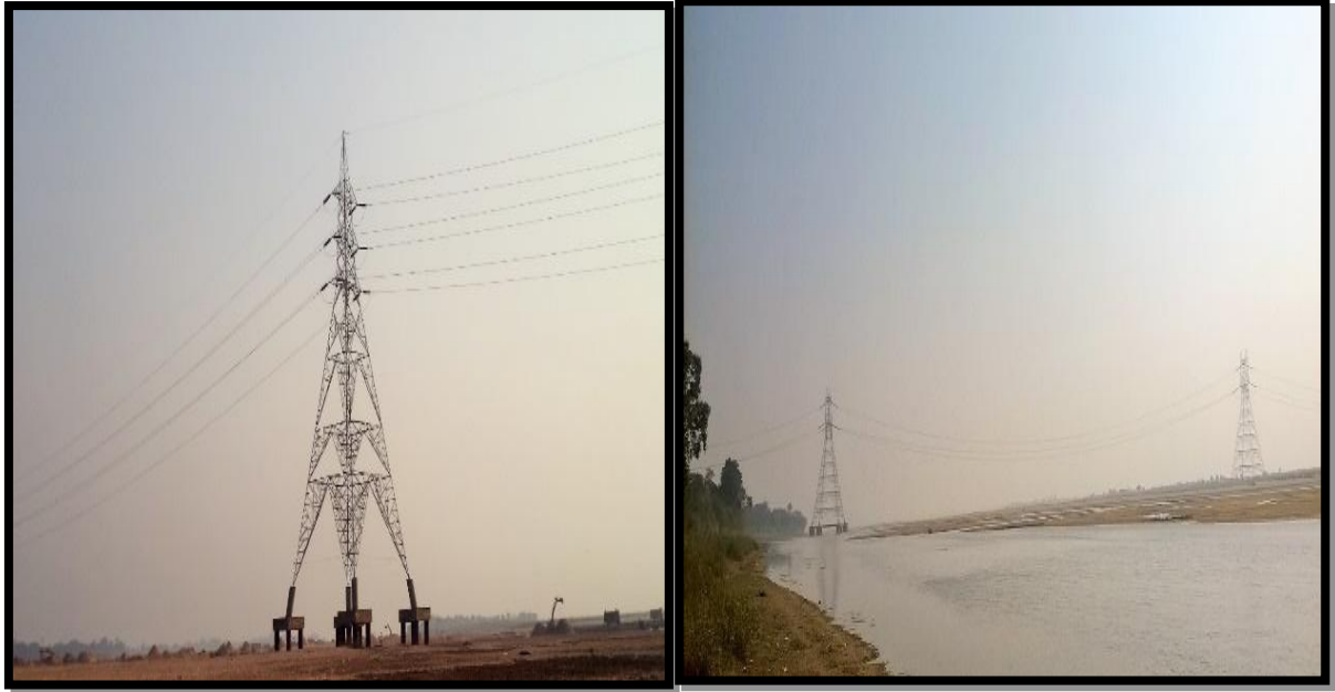
High tension line at Ch 103.3 km & Ch 116.07
