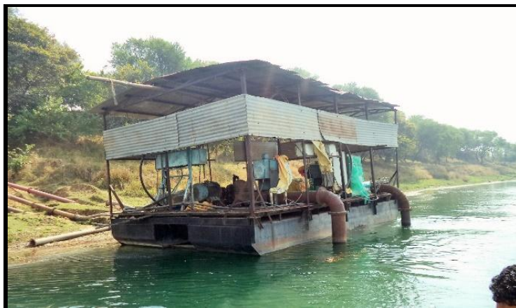
Water Pump at Ch 35.60 km
