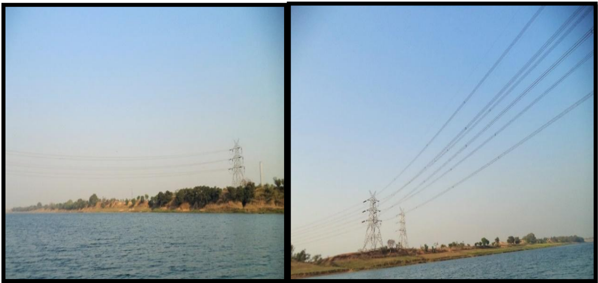
High tension line at Ch 28.41, 28.80 & 28.82 km
