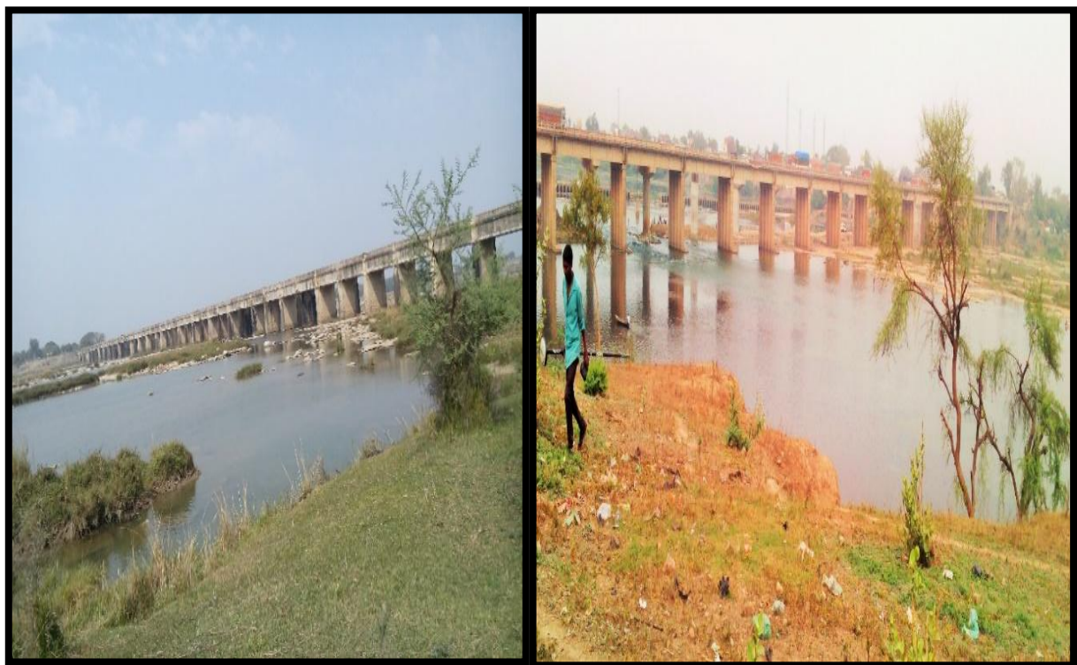
Gaughat Bridge at Ch 68.03 km&KM Chakghat Bridge and U/C Bridge at Ch 73.25 km
