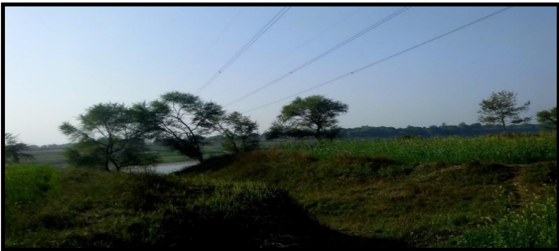
HT Line at Ch 18.17km
