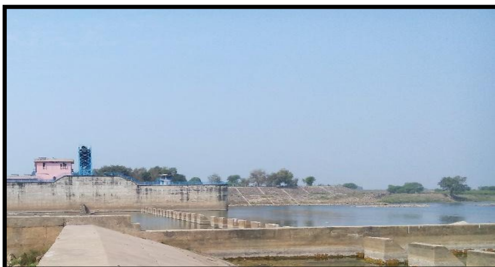
River Bank Pitch Protected at Ch 69.37 km
