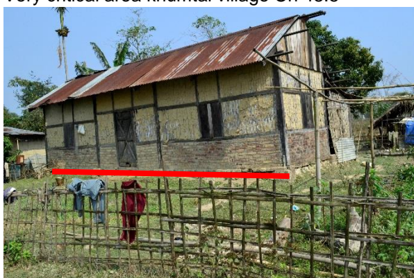
Flooding at the Moonsoon Period Red line Amola pathy Gaon
