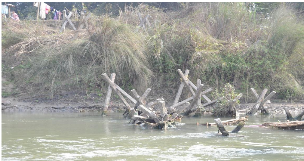
Figure 31 Unprotected, eroding bank of Dhansiri River ch 82.45
