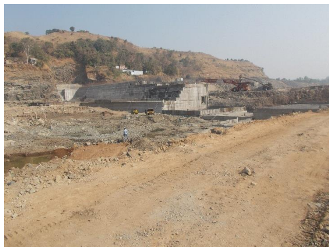
Weir at Garudeshwar
