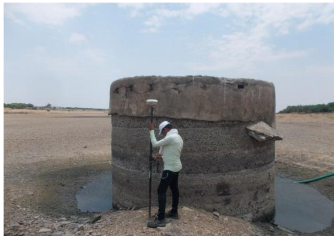
Figure 40 - Drinking Water Well
