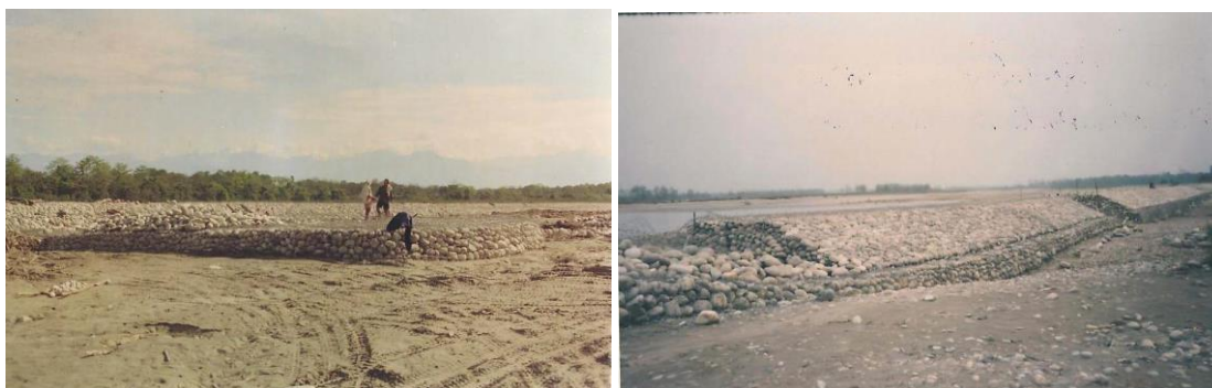
Figure 15 A deflector and plugging structure under construction near Suparna (Source: North Eastern Council (NEC) Evaluation of NEC funded projects in Arunachal Pradesh report)
