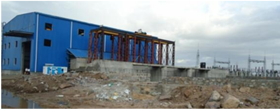
Figure 16 - Small Hydro Electric Plant (75.00 km Chainage)
