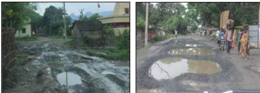
Figure 39: Severe damage inflicted due to heavy truck loads
