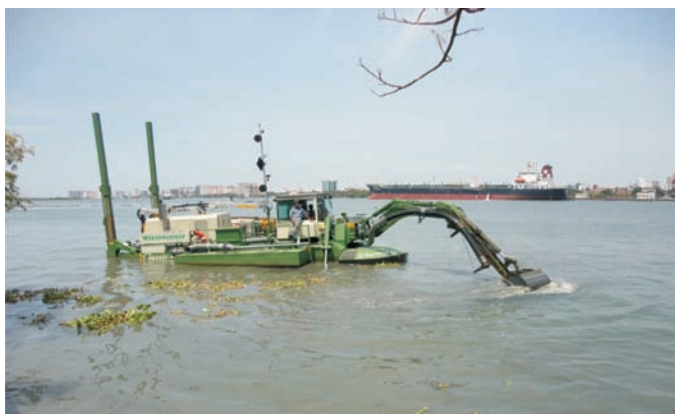
Amphibian Dredger "AD Manimala" under taking de-siltation works at Willington Island and Bolghatty Ro-Ro Jetty
