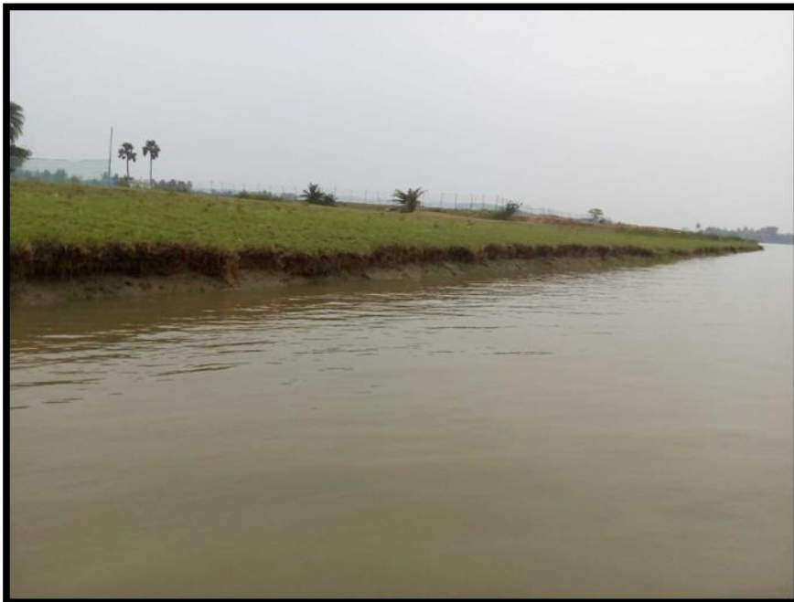
Soil Erosion at chainge 7.5
