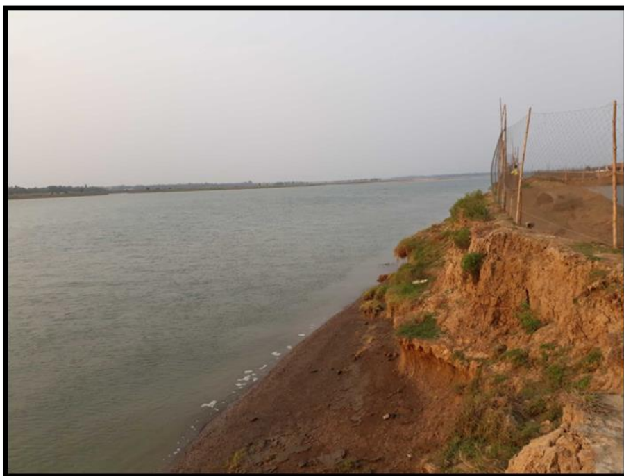
Unprotected Bank at Chainage 13.0
