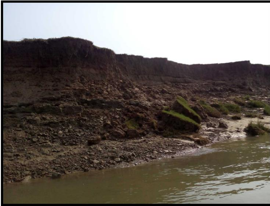
Soil Erosion at Chainge 11.0
