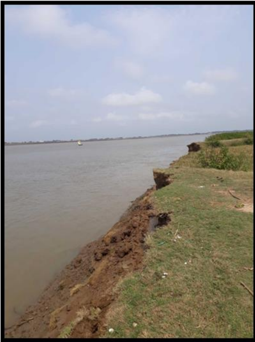
Bank Erosion at Chainage 13.0
