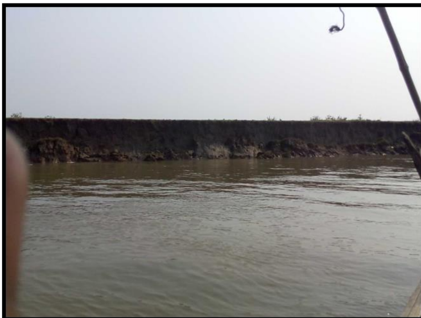
Unprotected Bank at chainge 6.0
