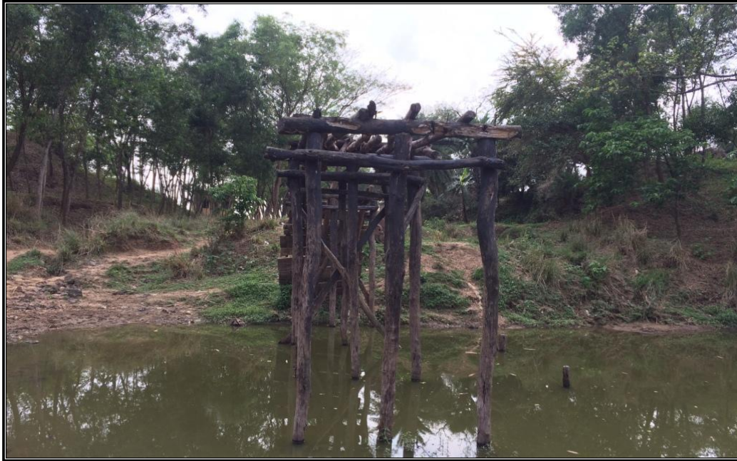
CHAINAGE 89.337 Km BROKEN WOODEN BRIDGE CHANCHAI
