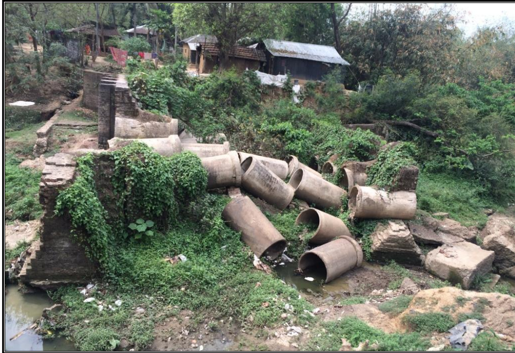
CHAINAGE 92.437 Km BROKEN CULVERT MAHESH DANGA
