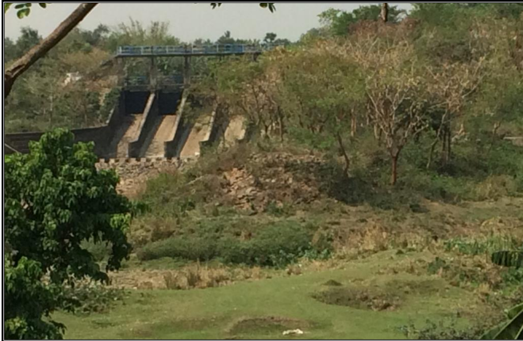
CHAINAGE 65.679 Km LOCK GATE KANCHAN NAGAR
