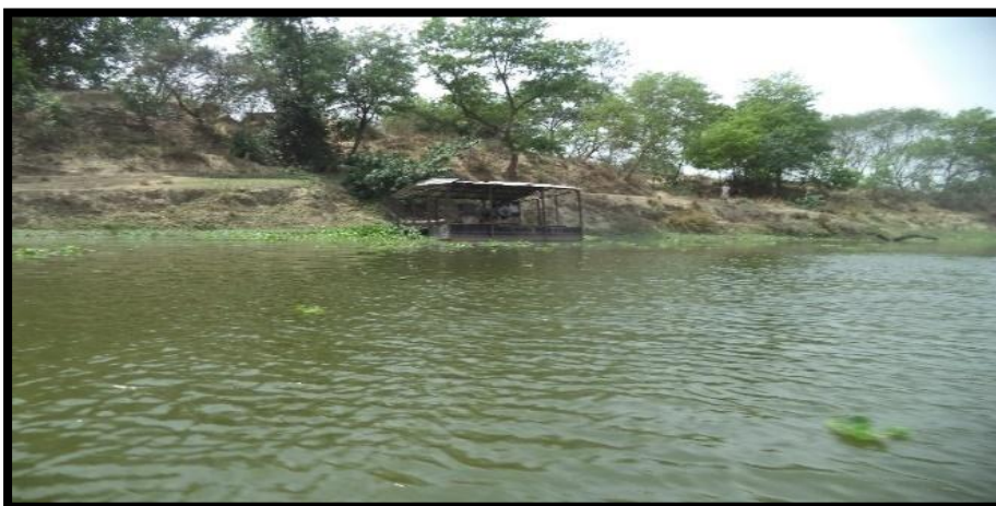
Water Pump at Ch 377.805 km
