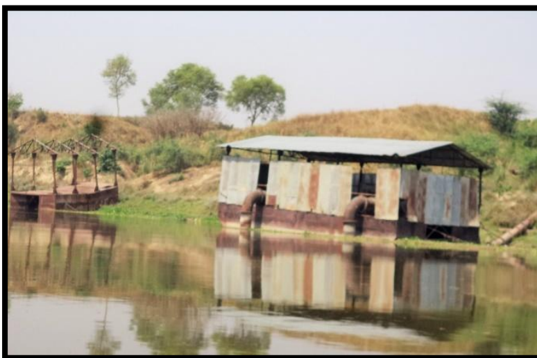
Water Pump at Ch 117.081 km
