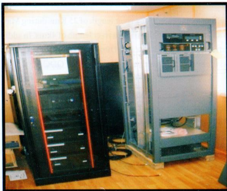
DGPS station –Control Room
