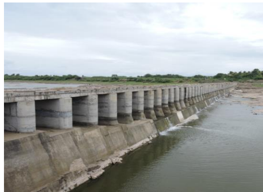
Figure 235 - Check Dam near Khedala Zunge village (ch. 1137.744km)
