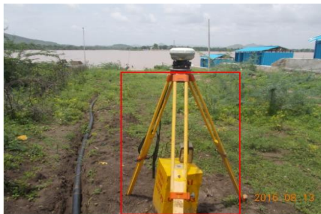
Benchmark pillar before flooding
