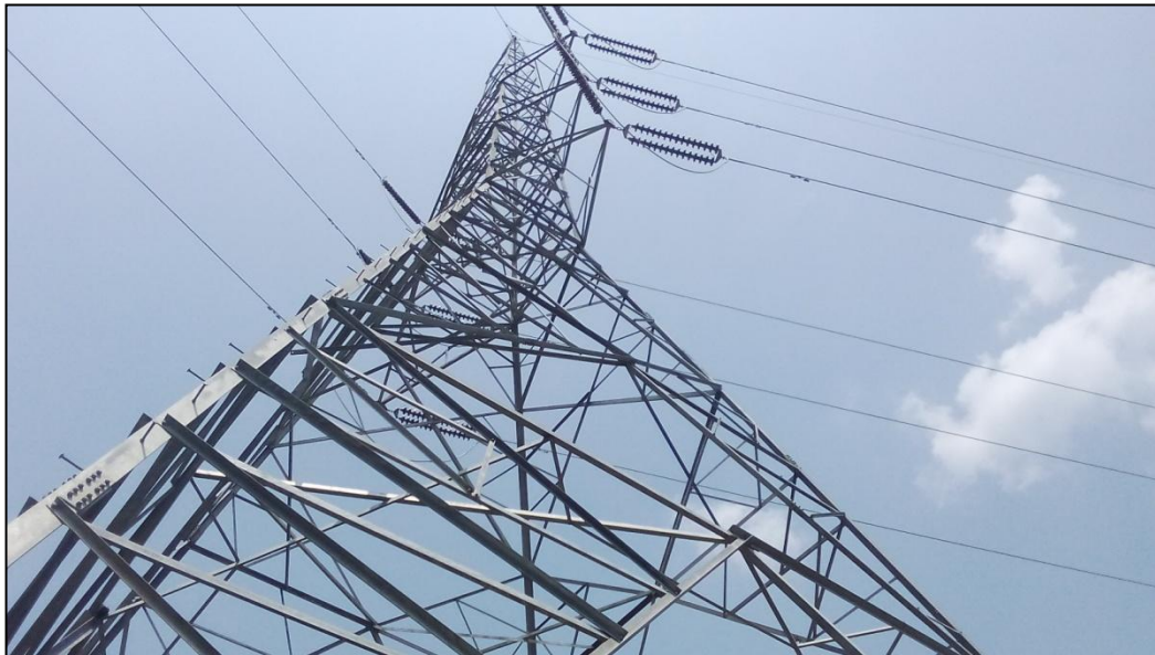
Figure 59-Electric Post (Chainage-15.348 km)
