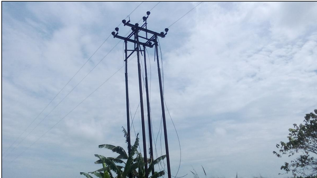
Figure 61- Electric Post near Chainage- 17.124 km
