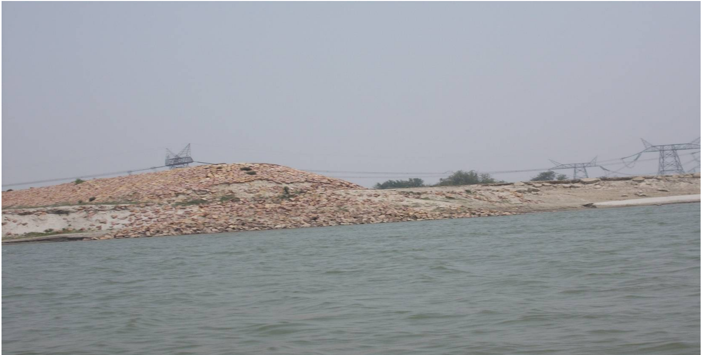
(Image: Spar Protection Collapse)
