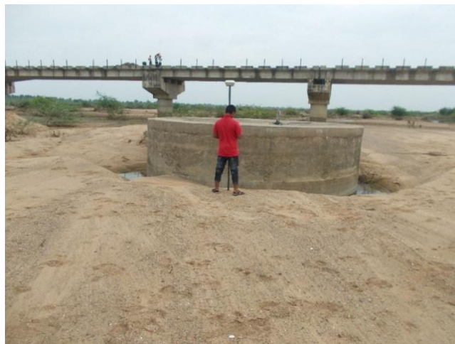
Figure 38 - Drinking Water Pump (6.5 km chainage) well on Manjira River
