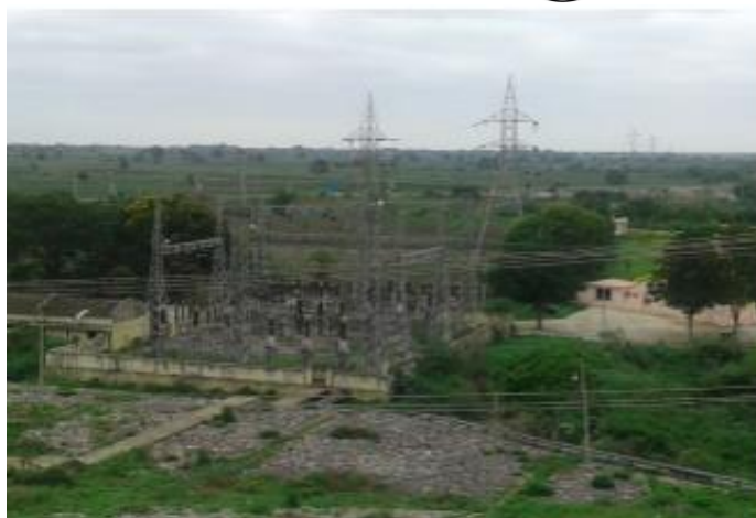
Figure 36 - The power sub-station near Singur Dam (245.0 km chainage)
