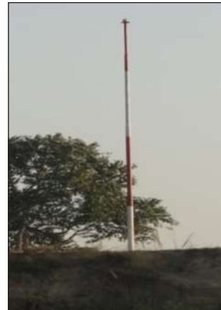
Light on Steel Pole
