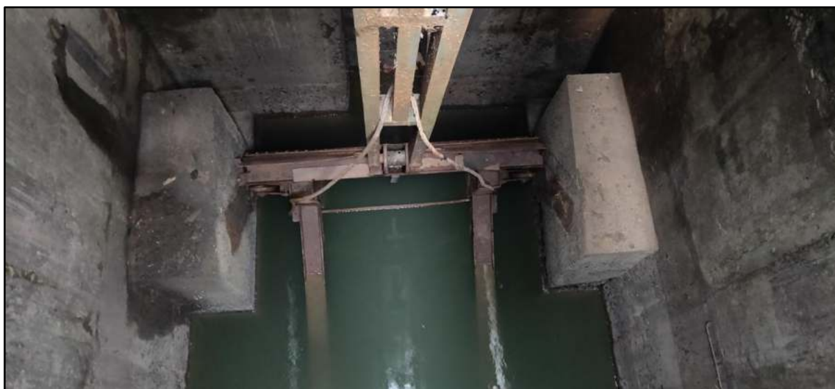
Figure 52: Lifting brackets and limb arms of Radial Gates
