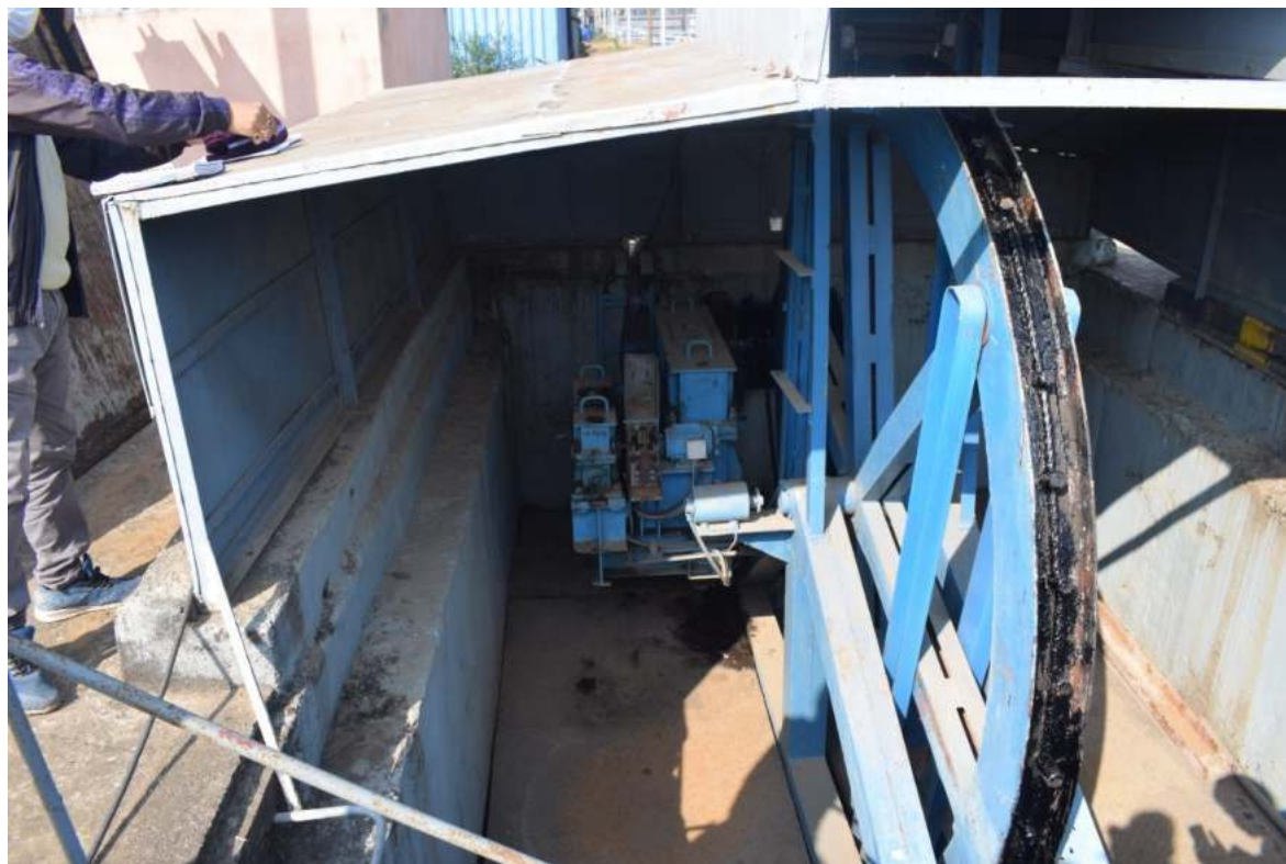
Figure 53: Operating System of Radial Gates
