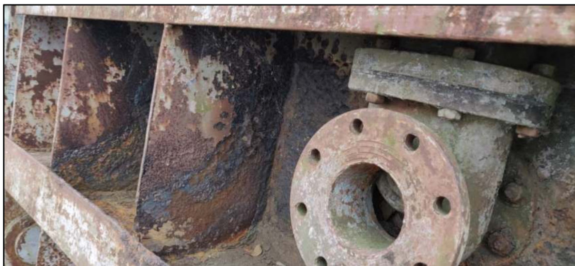
Figure 56: Deteriorated equalizing valve of Bulkhead Gates
