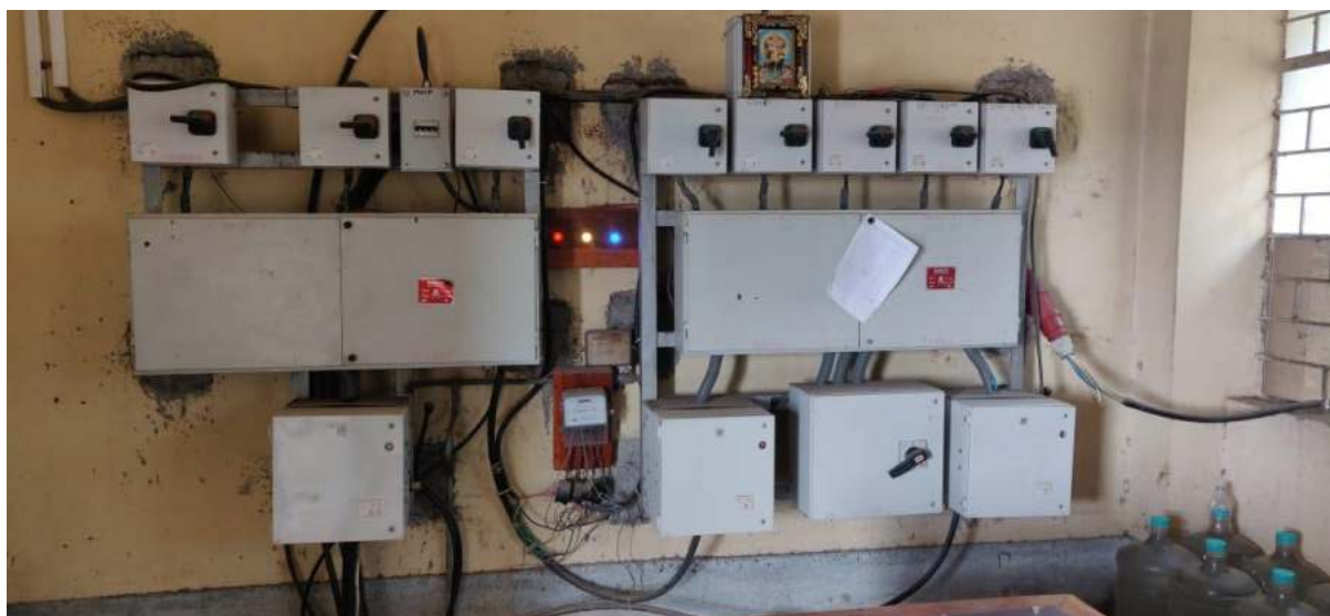
Figure 72: Electrical Control Room
