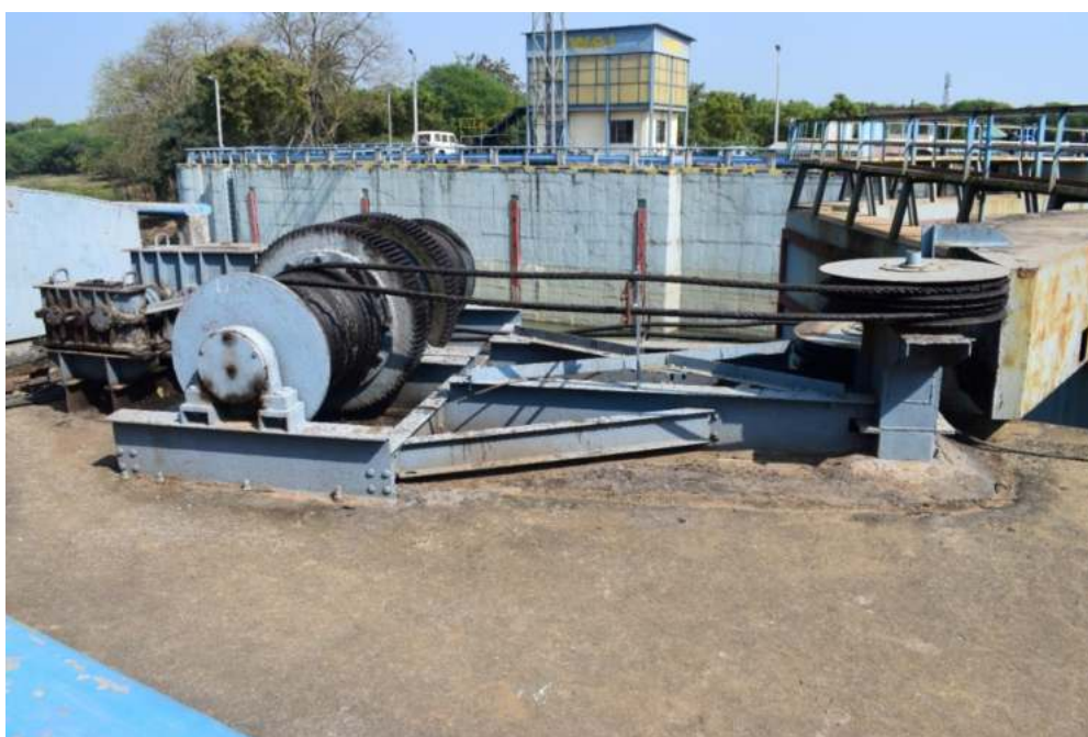
Figure 67: Temporary position indicator used to control gate opening
