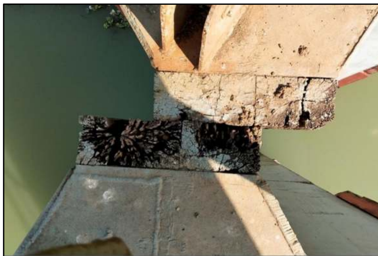
Figure 48: Condition of Seals of Mitre Gate of Farakka Lock
