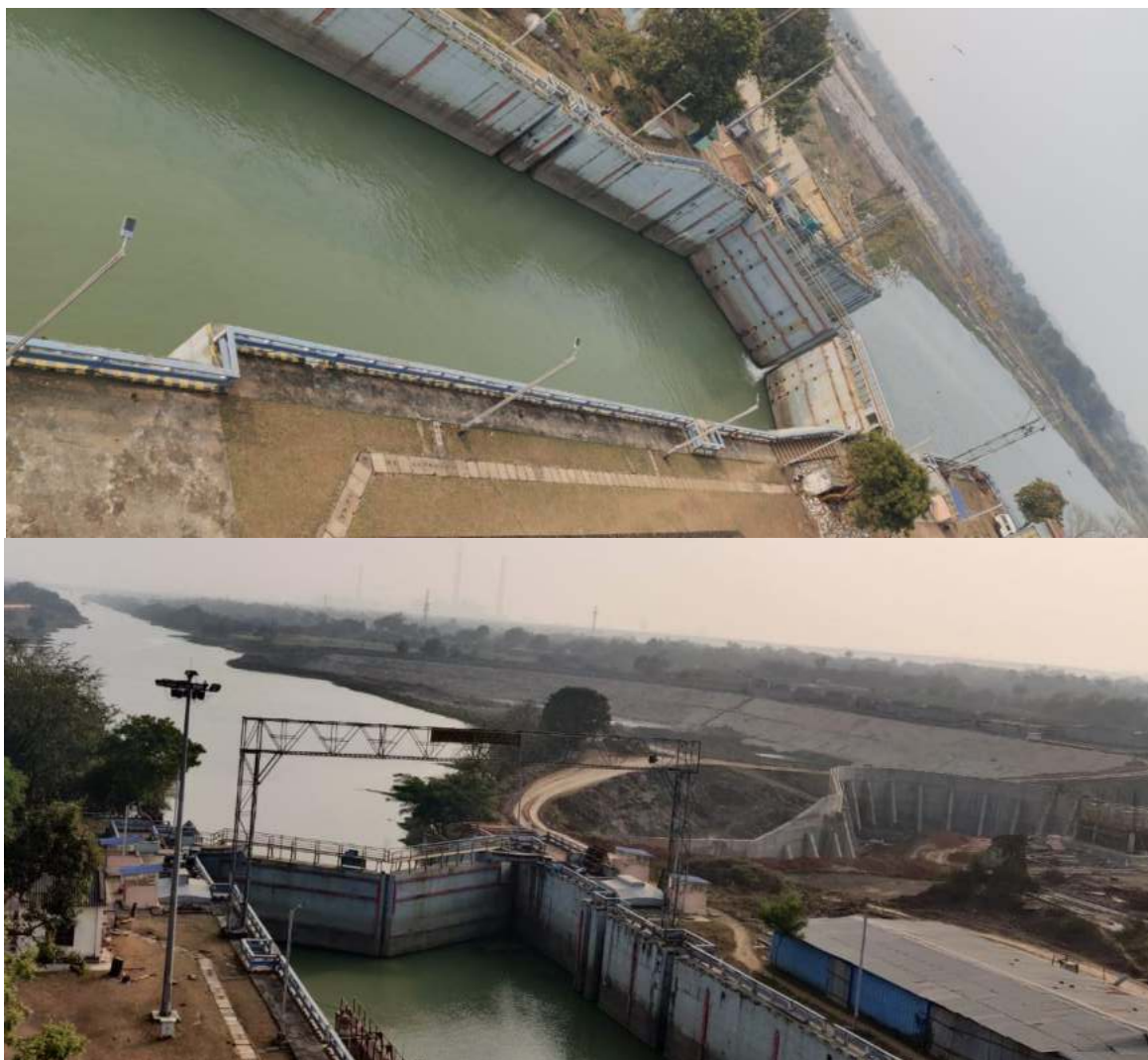
Figure 74: Lighting system at the lock site
