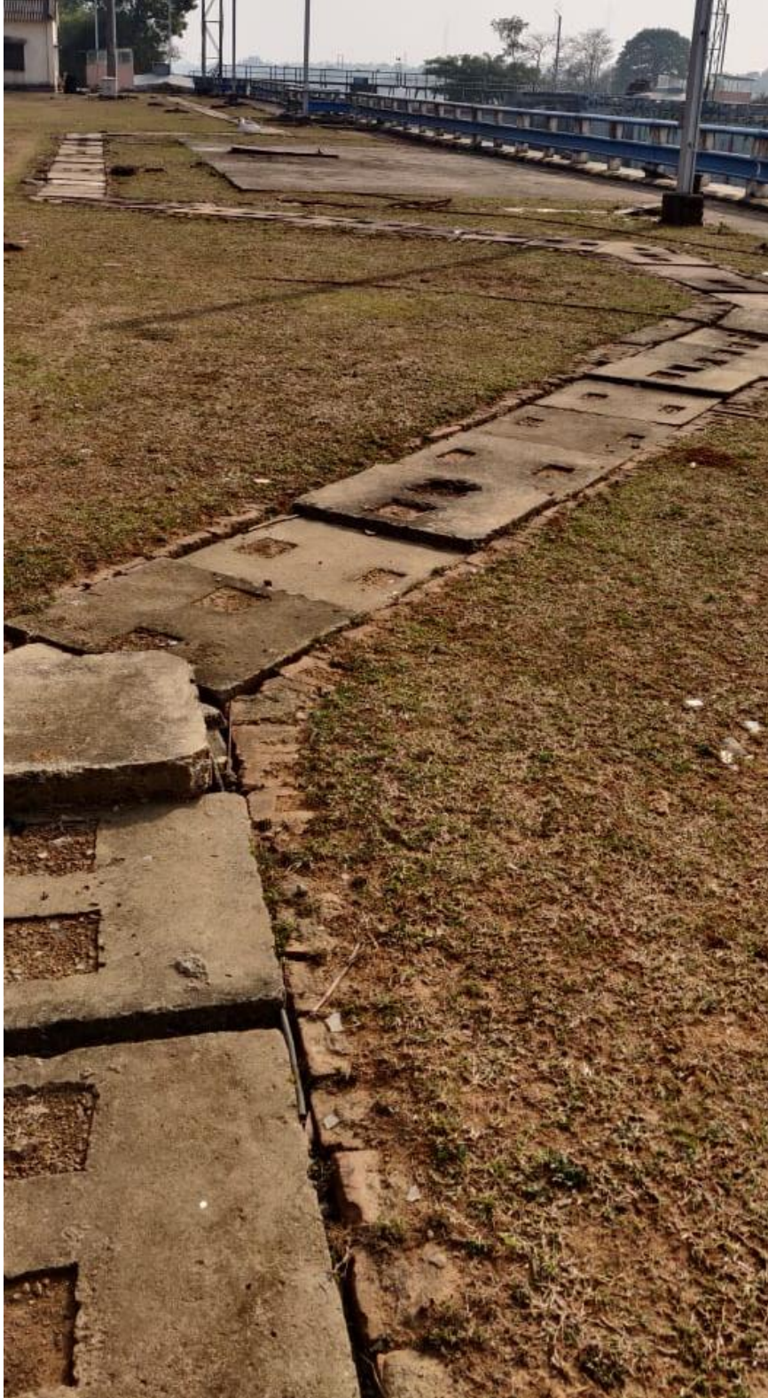
Figure 66: Cable trench for power cables
