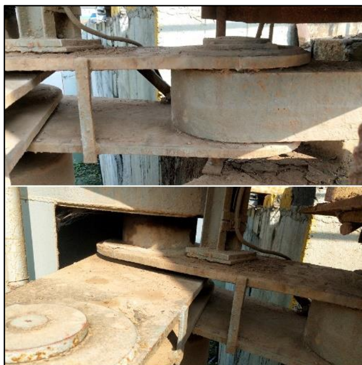
Figure 49: Top Bearing of Mitre Gates of Farakka Lock
