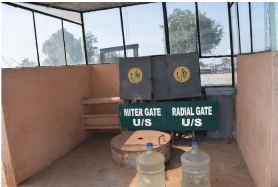
Figure 68: Local control system of u/s Mitre and Radial Gate
