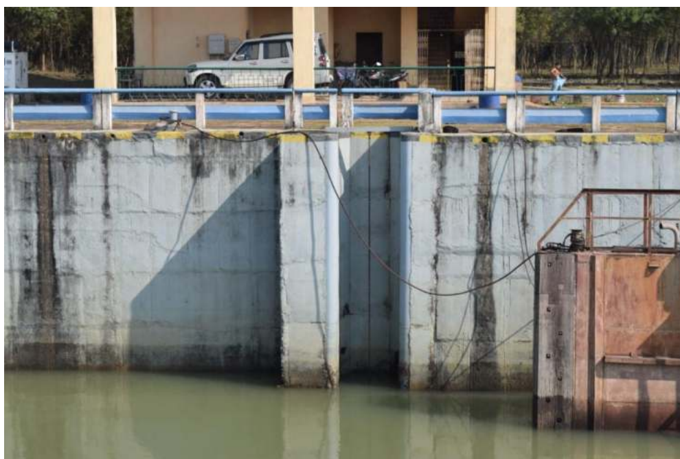
Figure 61: Damaged Fixed Type Bollard
