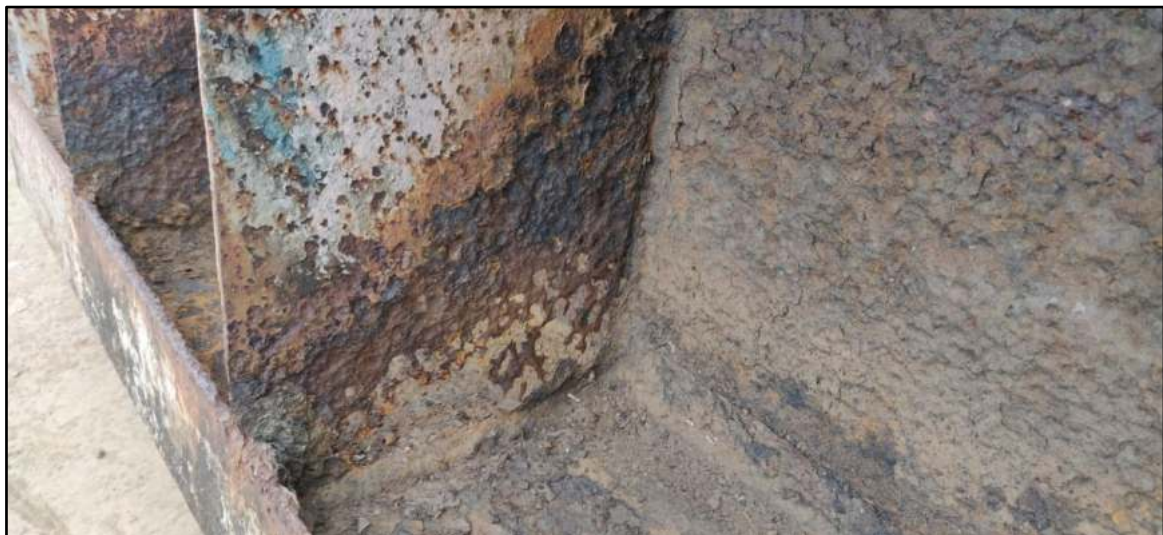
Figure 55: Heavy corrosion in Bulkhead Gates
