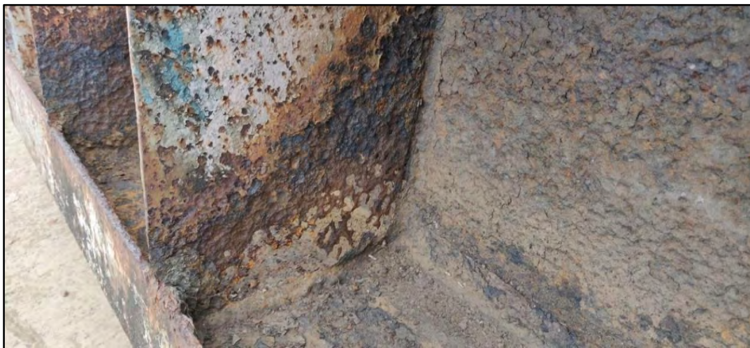
Figure 7.8 Heavy corrosion in Bulkhead Gates
