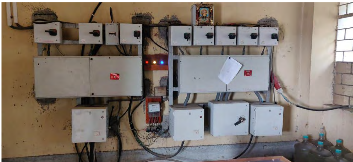
Figure 8.3 Electrical Control Room
