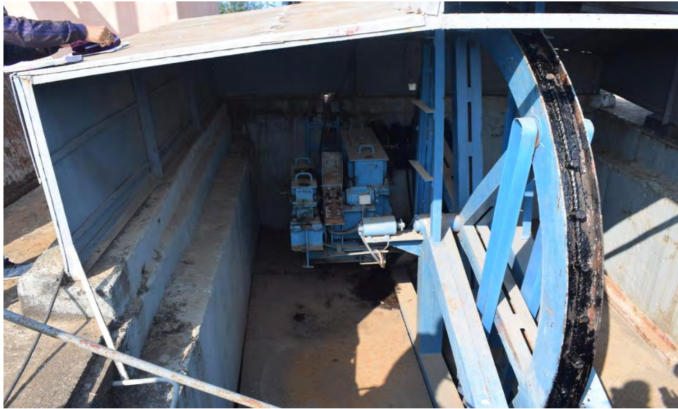
Figure 7.6 Operating System of Radial Gates
