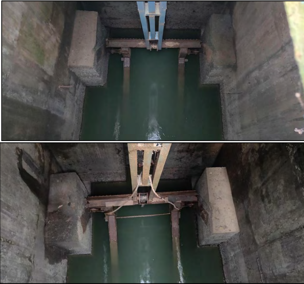
Figure 7.5 Lifting brackets and limb arms of Radial Gates
