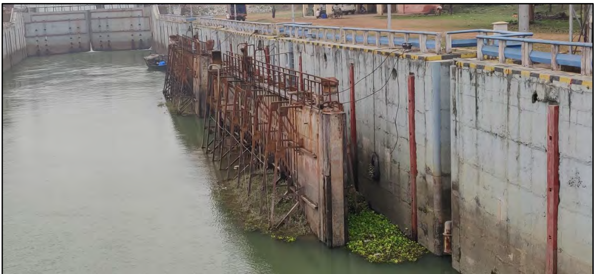
Figure 7.11 Caisson Gates for Mitre Gate Maintenance at Farakka Lock
