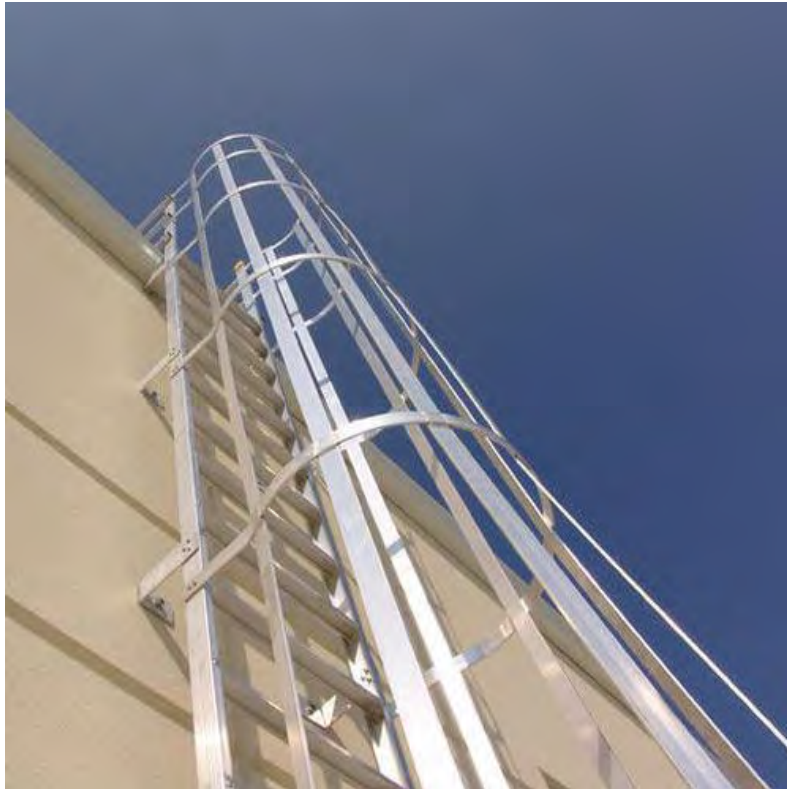
Figure 5.15 A picture of vertical access ladders with round safety tunnel
