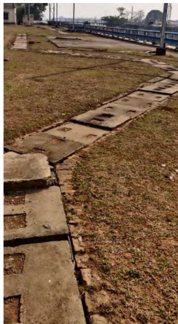
Figure 5.14 Electrical cable trench
