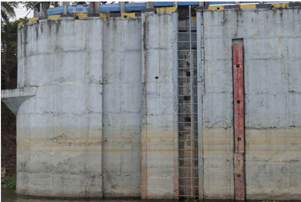
Figure 5.7 Fixed water level gauge in ladder recess
