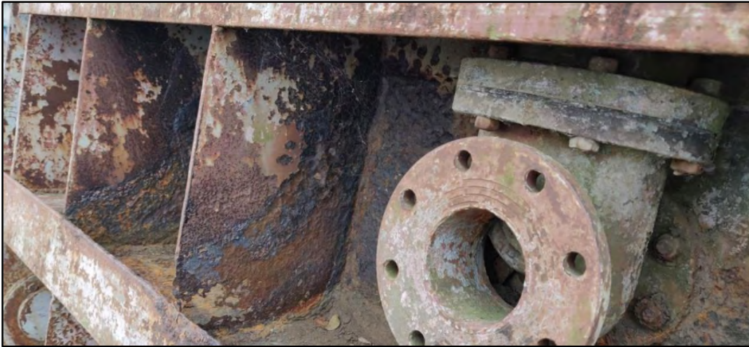
Figure 7.9 Deteriorated equalizing valve of Bulkhead Gates
