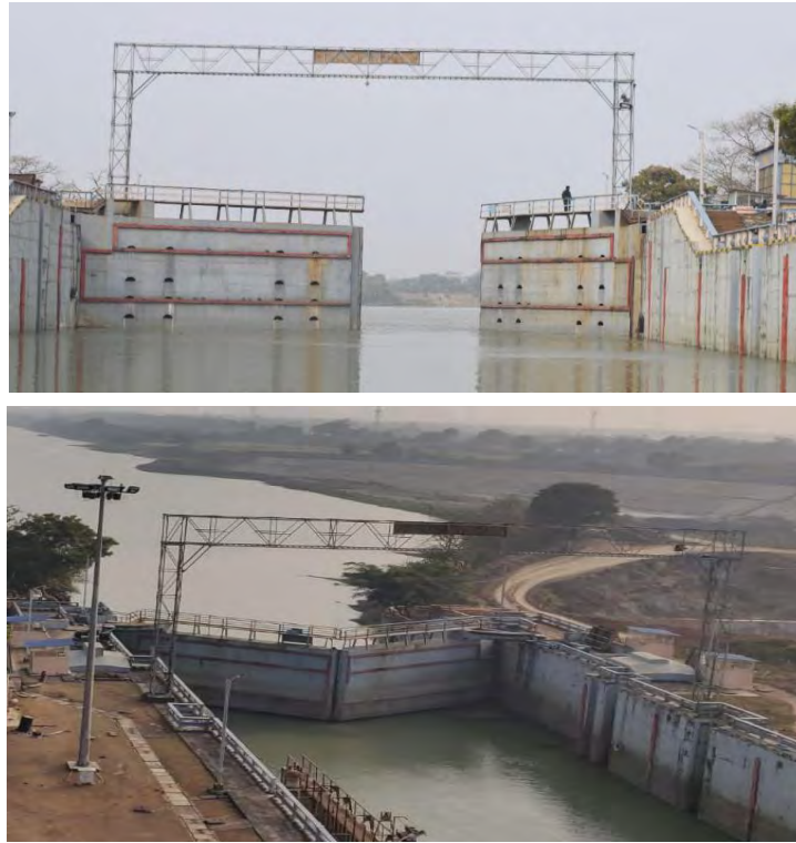
Figure 5.13 Steel lattice type cable bridges
