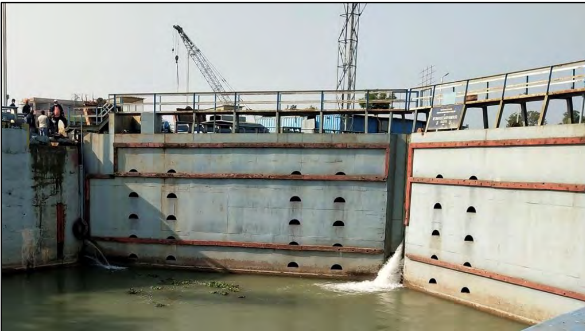
Figure 7.1 Mitre Gates of Farakka Lock
