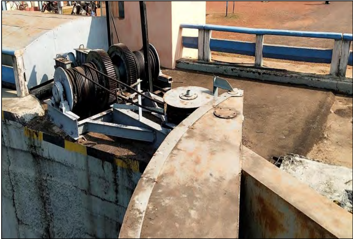
Figure 7.4 Operating Mechanism of Mitre Gates of Farakka Lock
