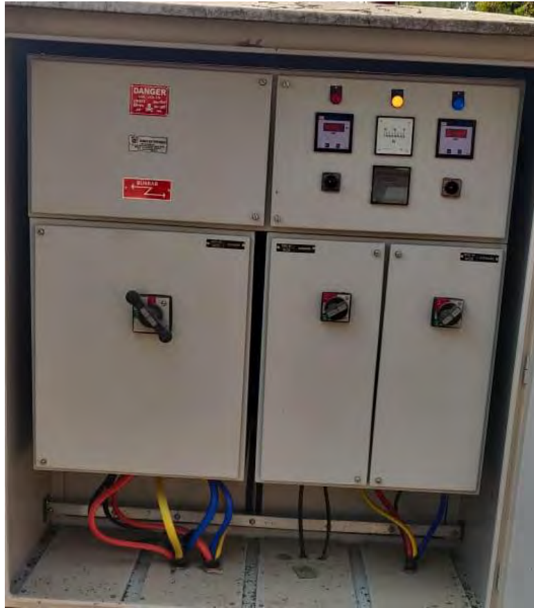
Figure 8.2 Electrical sub-station distribution board
