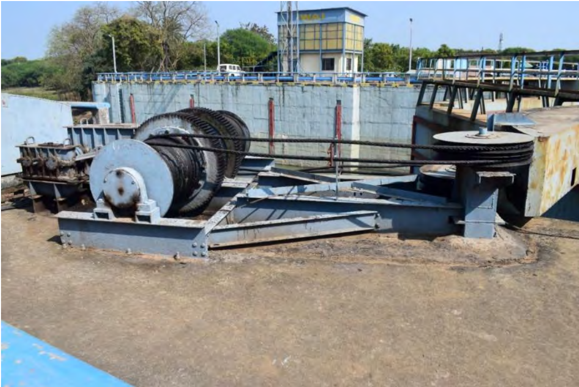
Figure 8.4 Temporary position indicator used to control gate opening
