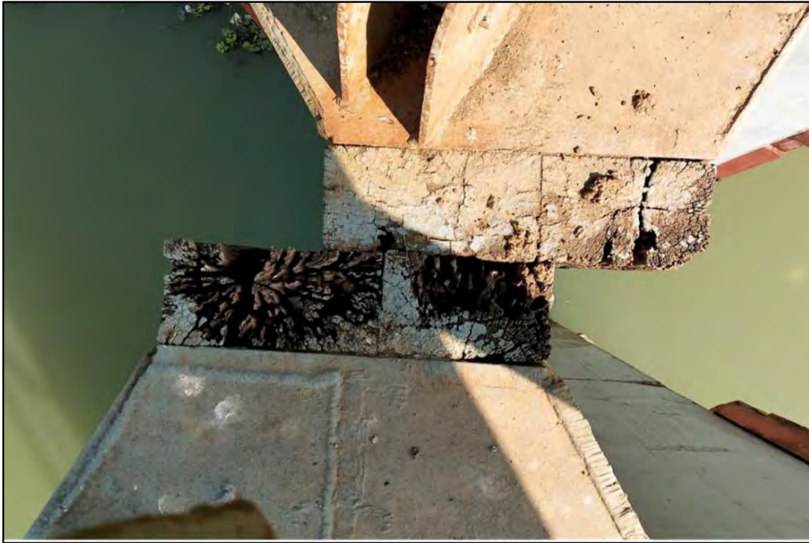
Figure 7.2 Condition of Seals of Mitre Gate of Farakka Lock
