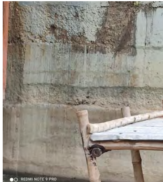
Figure 5.6 Guide Walls Damaged – Honey Combing & Cracks
