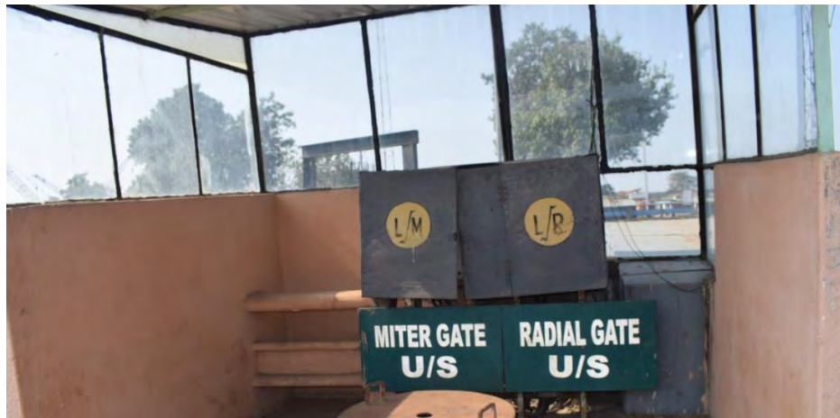
Figure 8.5 Local control system of u/s Mitre and Radial Gate
