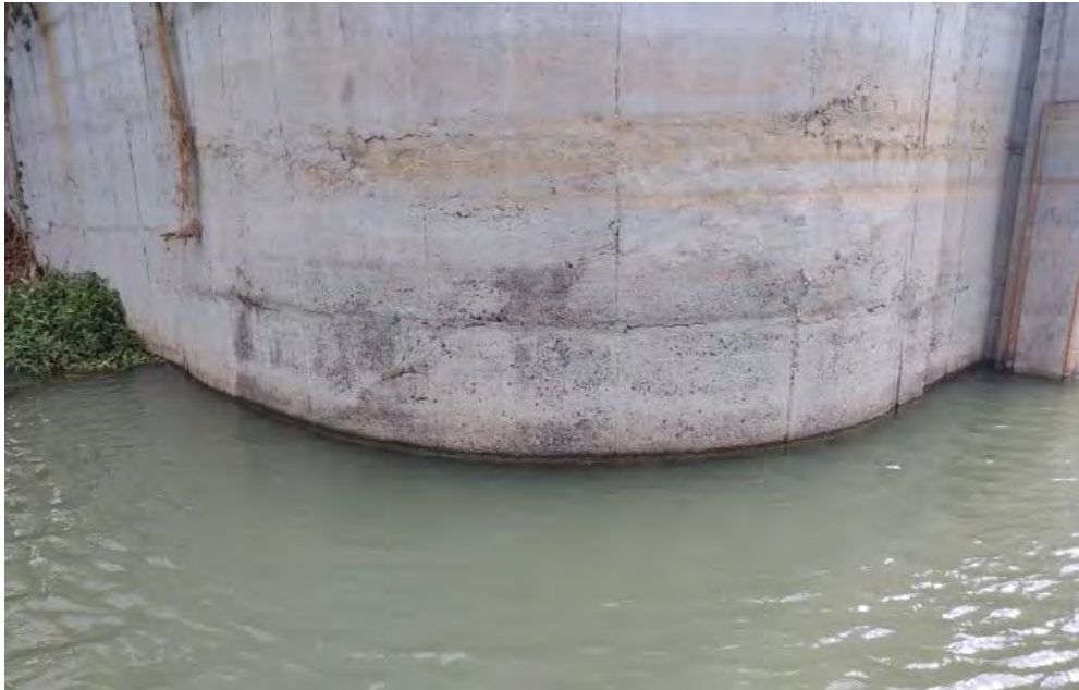
Figure 5.5 Guide Walls Damaged & Vegetation
