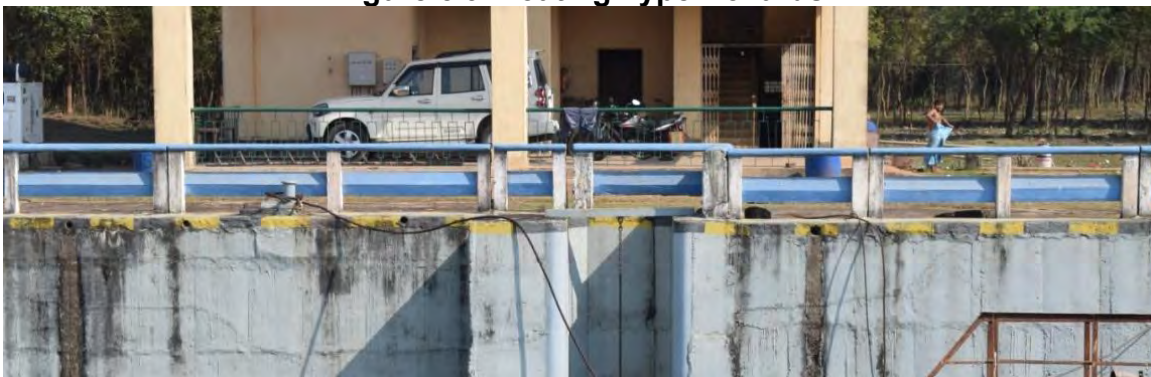
Figure 5.10 Damaged Fixed Type Bollard
