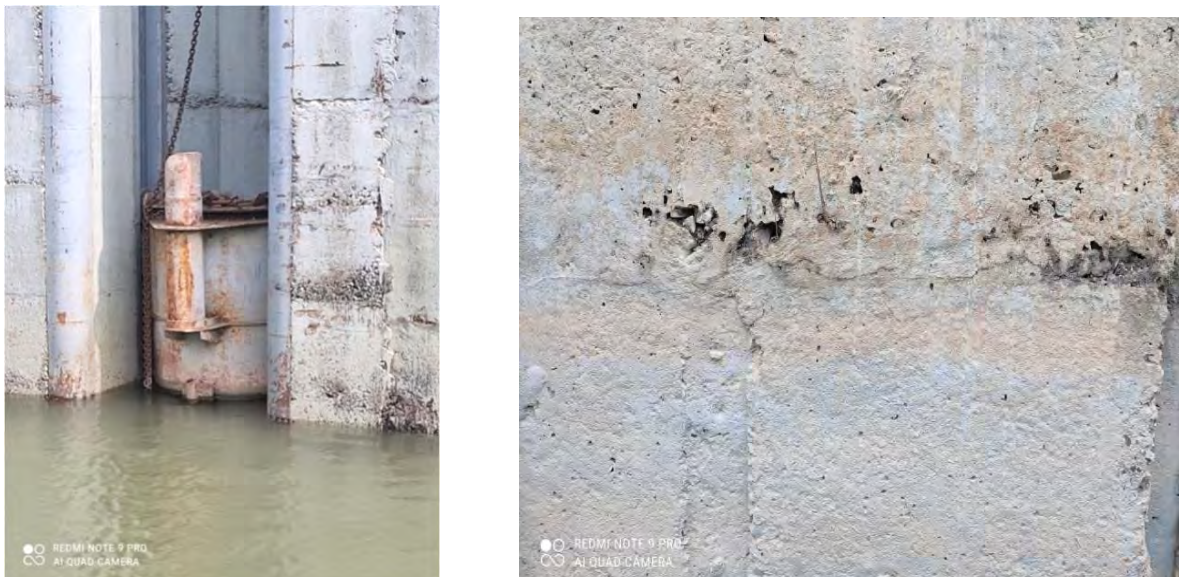
Figure 5.3 Lock Chamber side walls damaged
