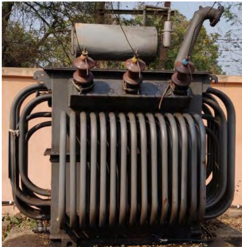
Figure 8.1 A 11 kV to 415 V Transformer
