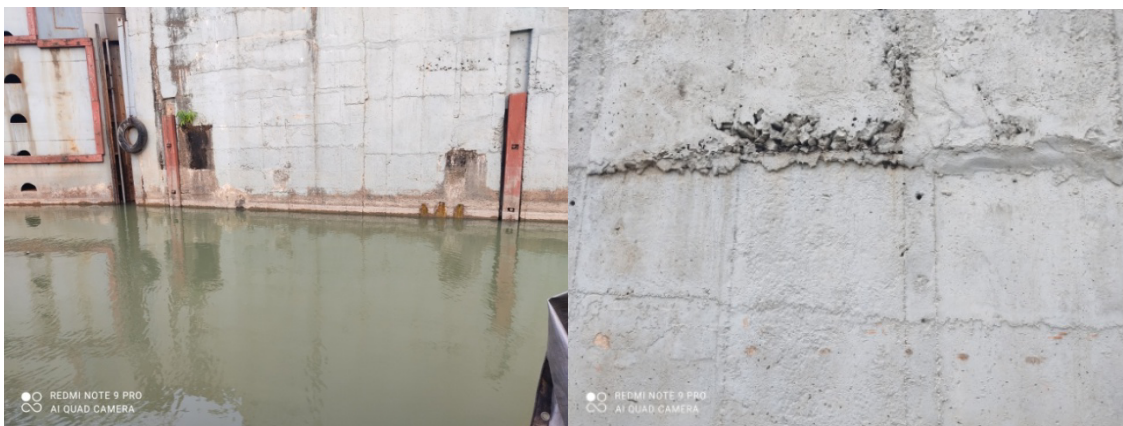
Figure 4.46 Honey Combing in Lock Walls
