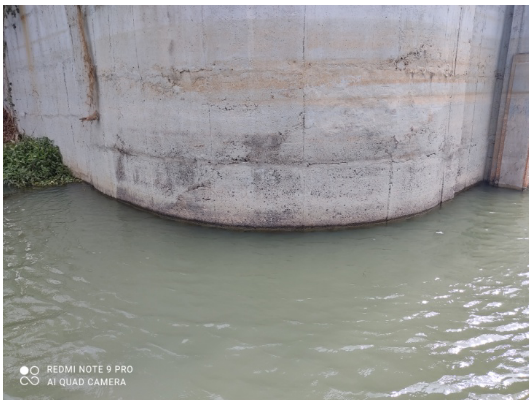
Figure 4.79 Guide Walls Damaged & Vegetation
