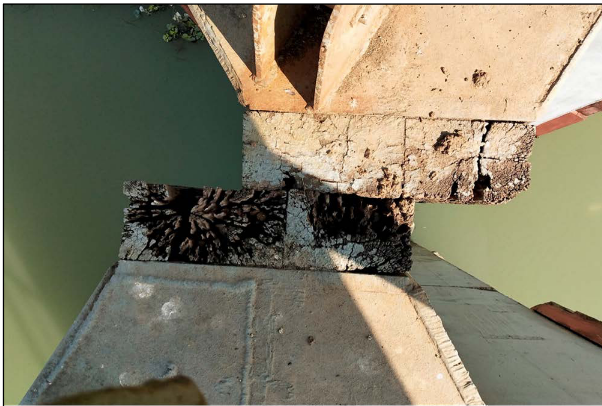
Figure 4.5 Condition of Seals of Mitre Gate of Farakka Lock
