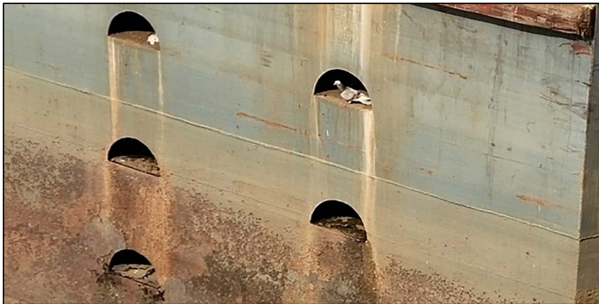
Figure 4.4 Corrosion of Submerged Section of Mitre Gates of Farakka Lock
