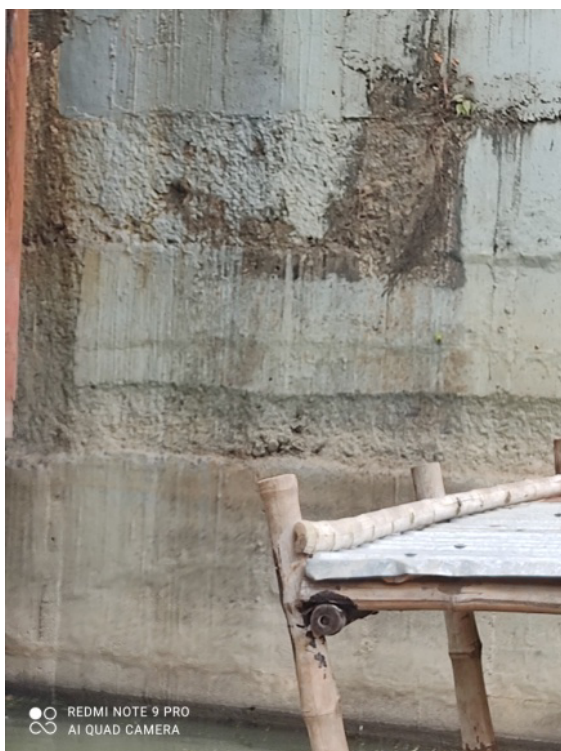
Figure 4.20 Guide Walls Damaged – Honey Combing & Cracks
