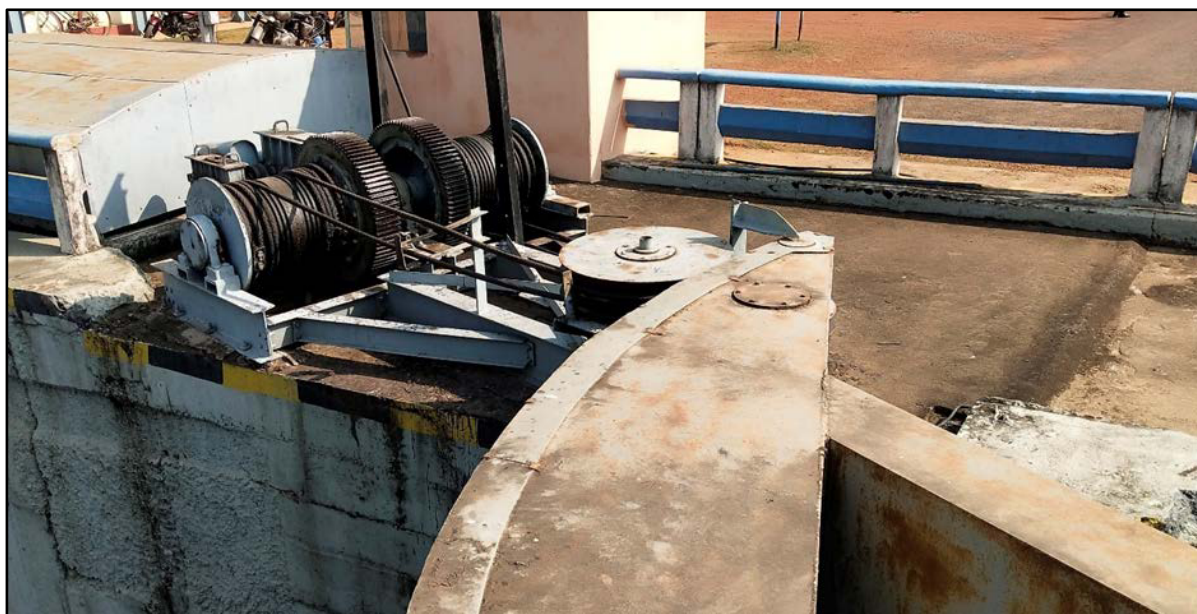
Figure 4.7 Operating Mechanism of Mitre Gates of Farakka Lock
