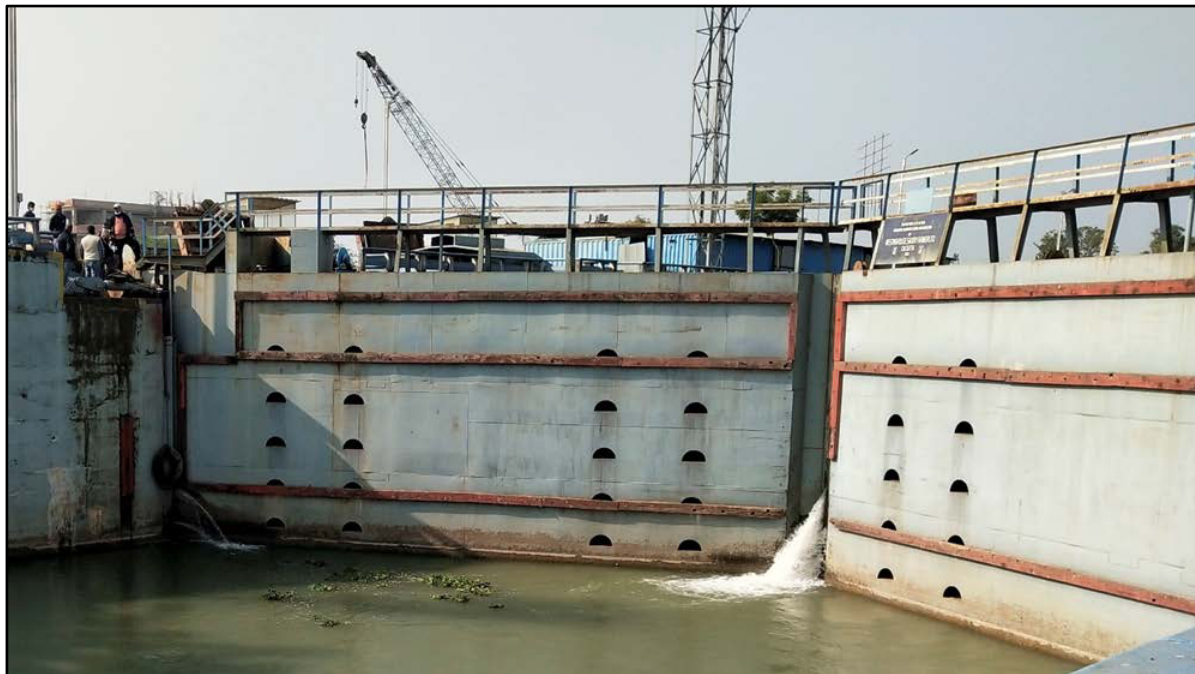
Figure 4.2 Mitre Gates of Farakka Lock
