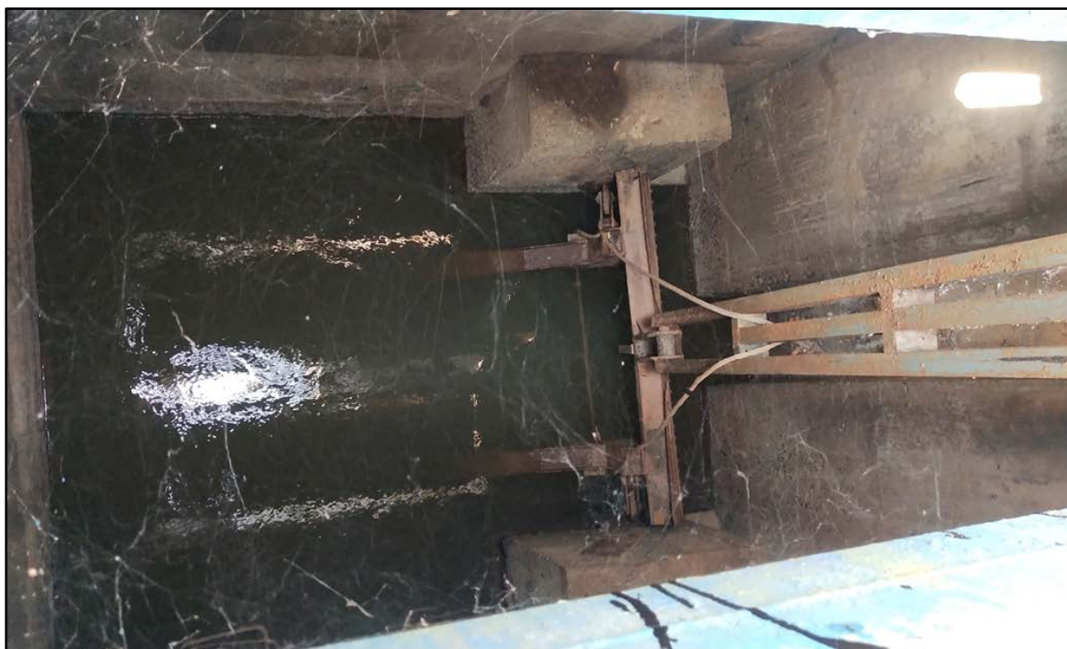
Figure 4.10 Lifting brackets and limb arms of Radial Gates
