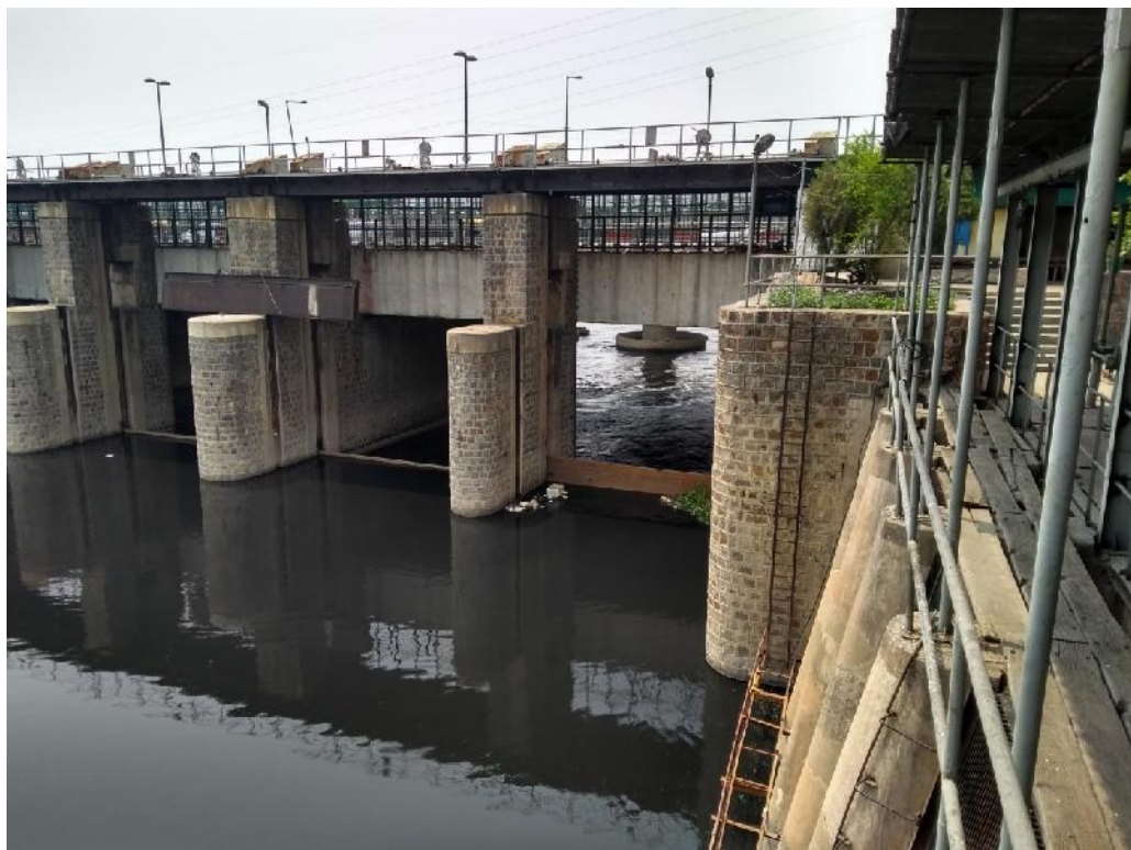
Fig. 2.32 Existing Condition of Gates at Yamuna Barrage ITO, Delhi
