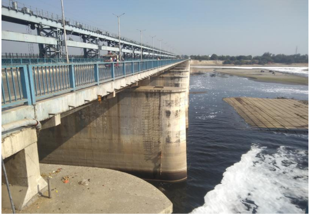
Fig. 2.42 Present View of Gates and piers from downstream of Gokul Barrage at CH 842 KM
