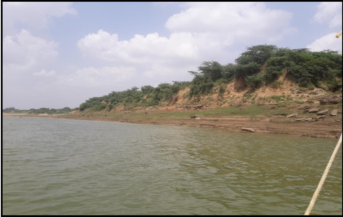
Fig No. 28 Steep cut Right side CH 42.700 km
