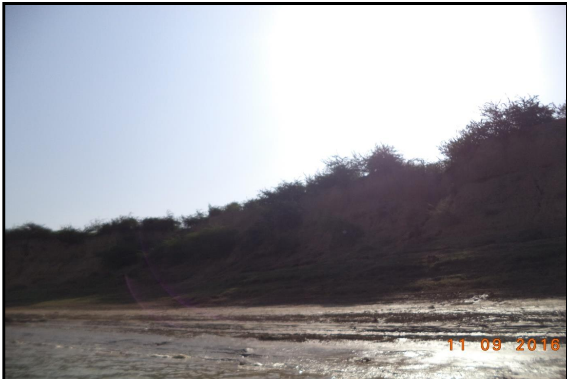
Fig No. 25 Steep cut Right side CH 27.000 km
