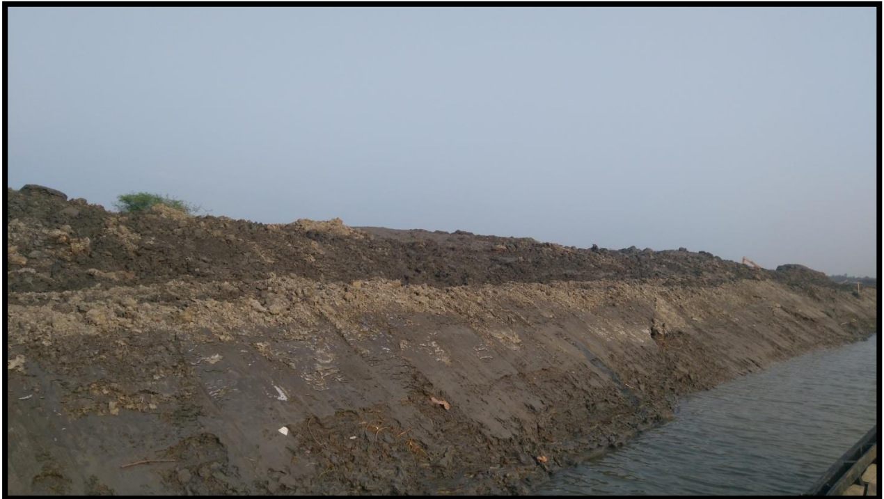
RIGHT BANK AT CHAINAGE 37
