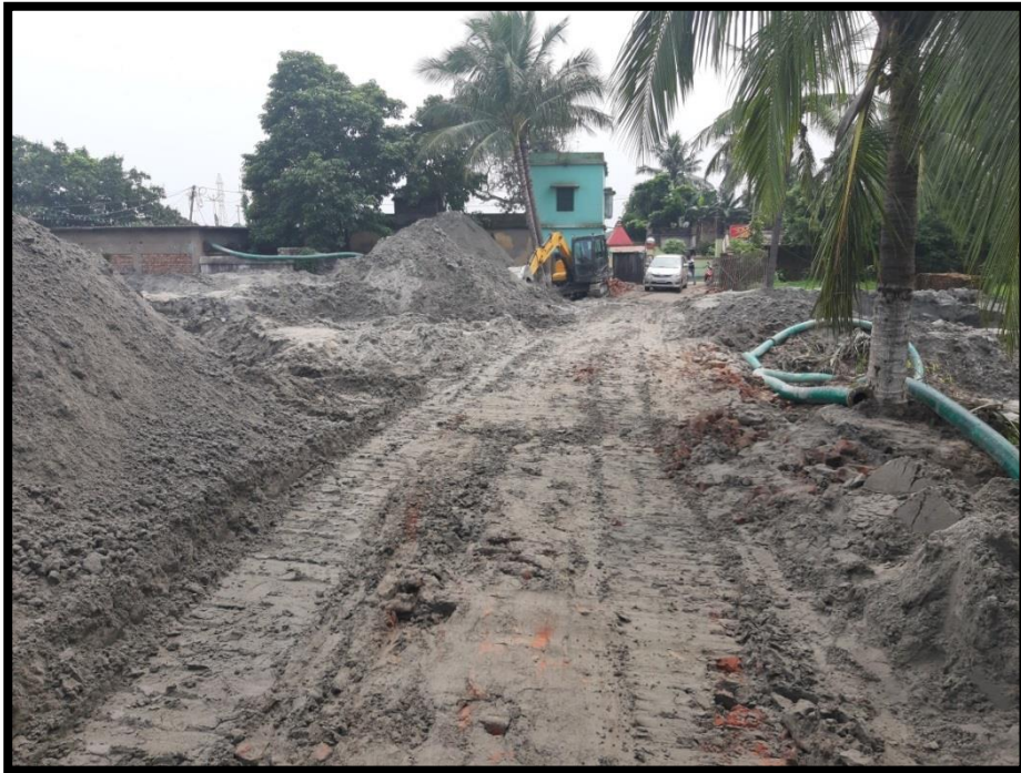
Land acquired by M/s River Waterlink Pvt. Ltd. for RO-RO operations (Pic-1)
