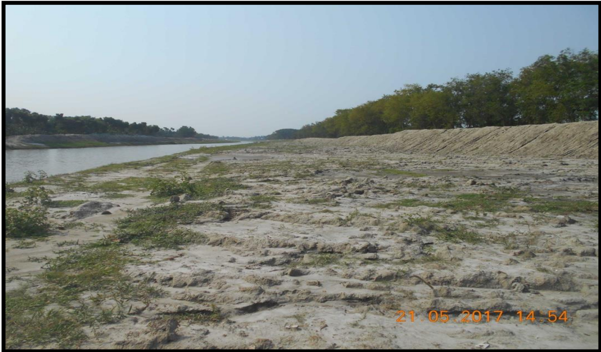
RIGHT BANK AT CHAINAGE 49.4
