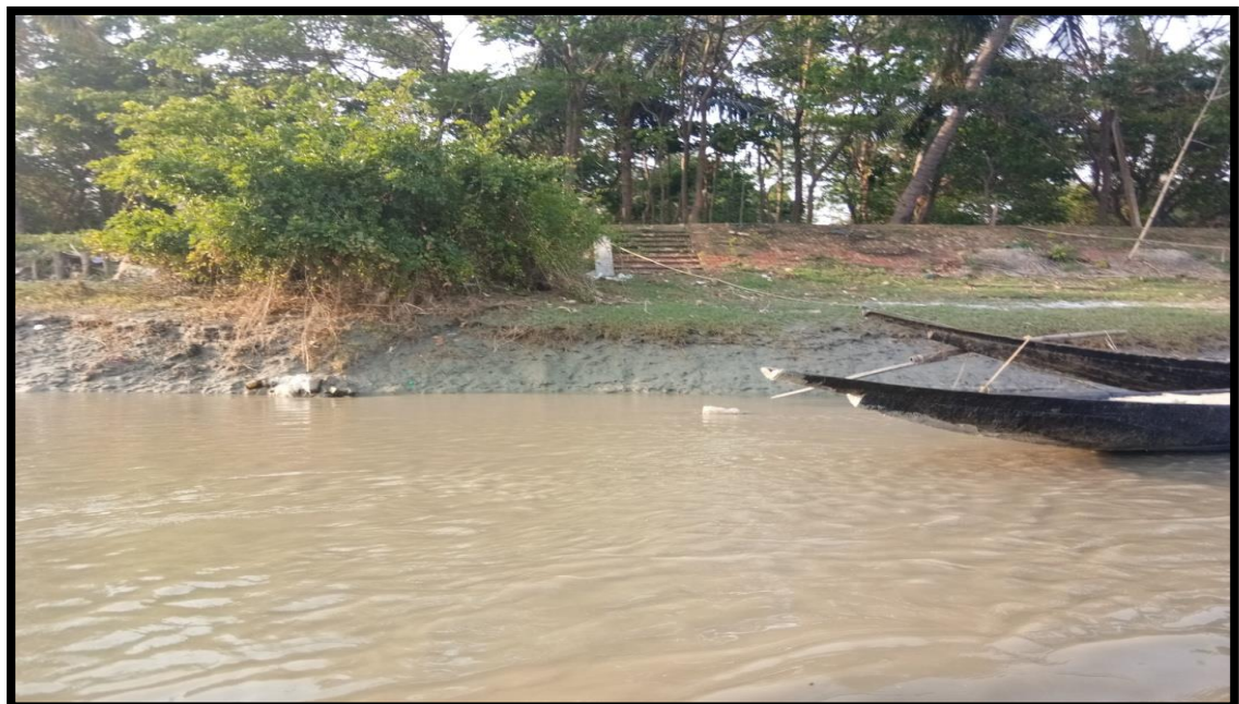
RIGHT BANK AT CHAINAGE 17.4
