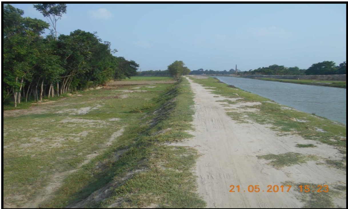
RIGHT BANK AT CHAINAGE 50
