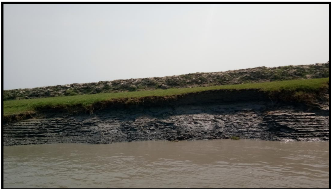
RIGHT BANK AT CHAINAGE 12
