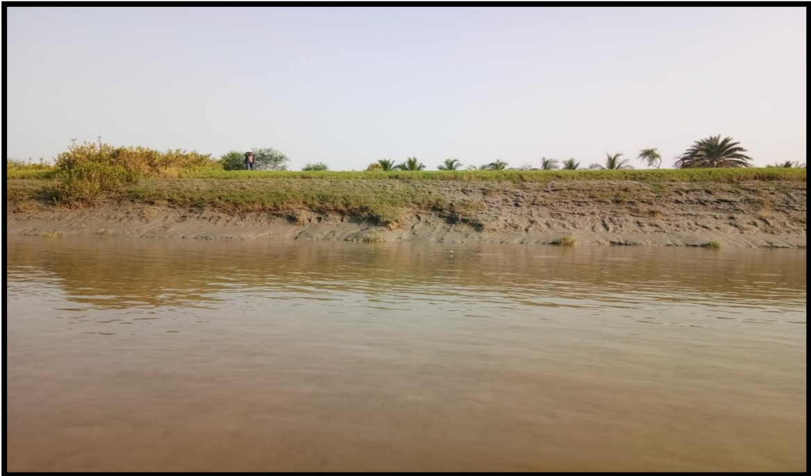
RIGHT BANK AT CHAINAGE 15.1
