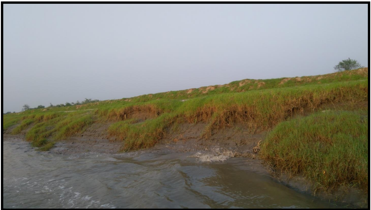
RIGHT BANK AT CHAINAGE 33
