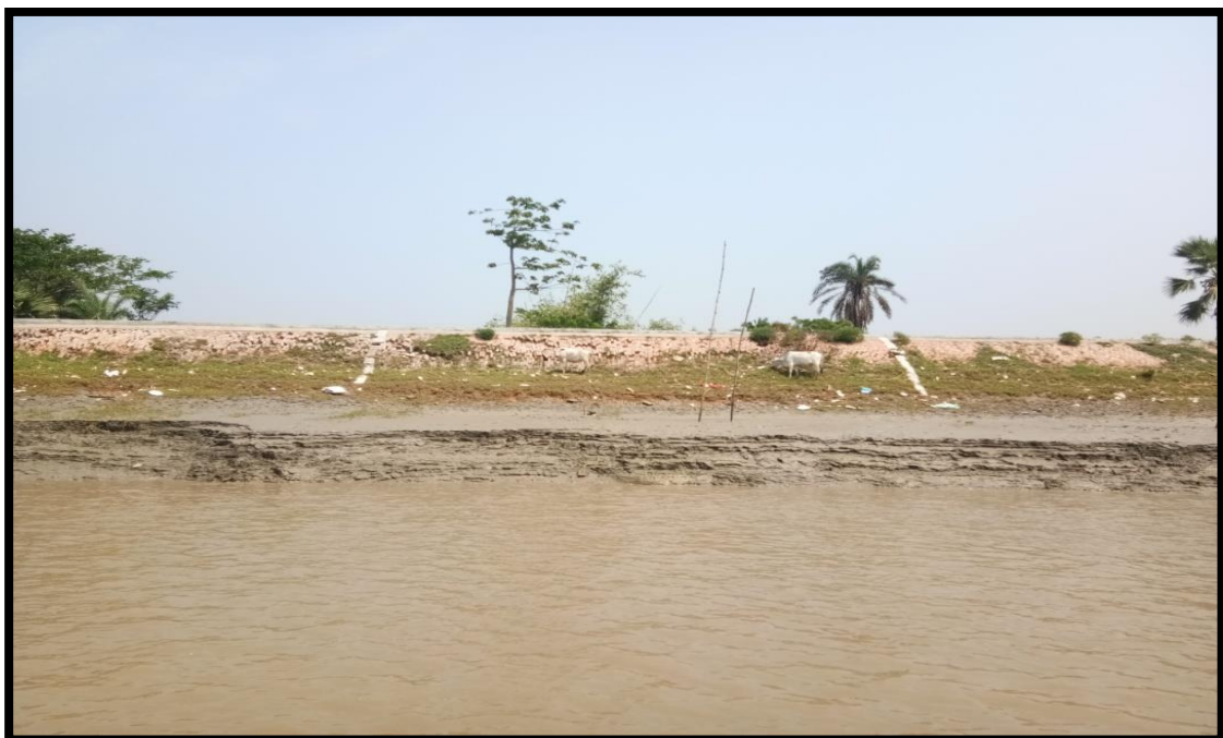
RIGHT BANK AT CHAINAGE 12.4
