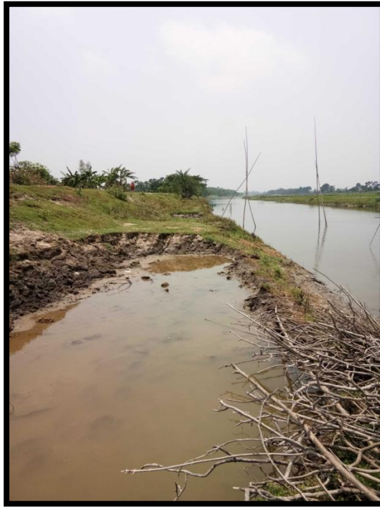
RIGHT BANK AT CHAINAGE 61.5
