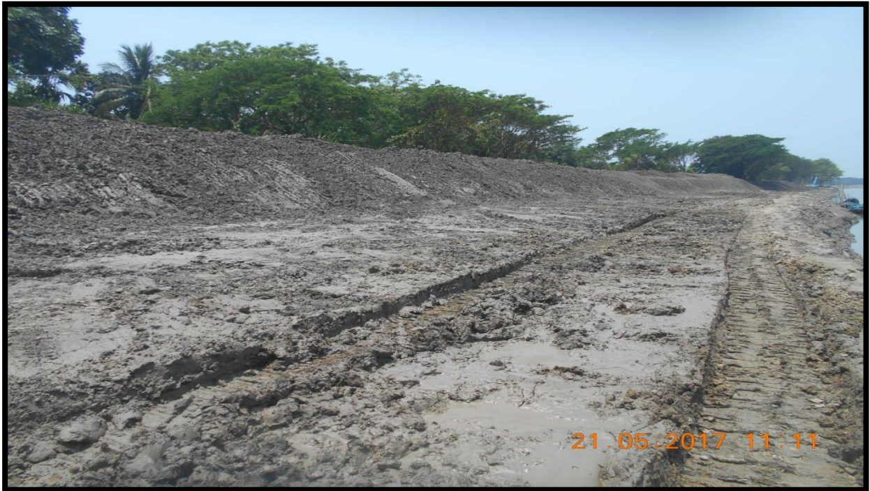
RIGHT BANK AT CHAINAGE 47.9
