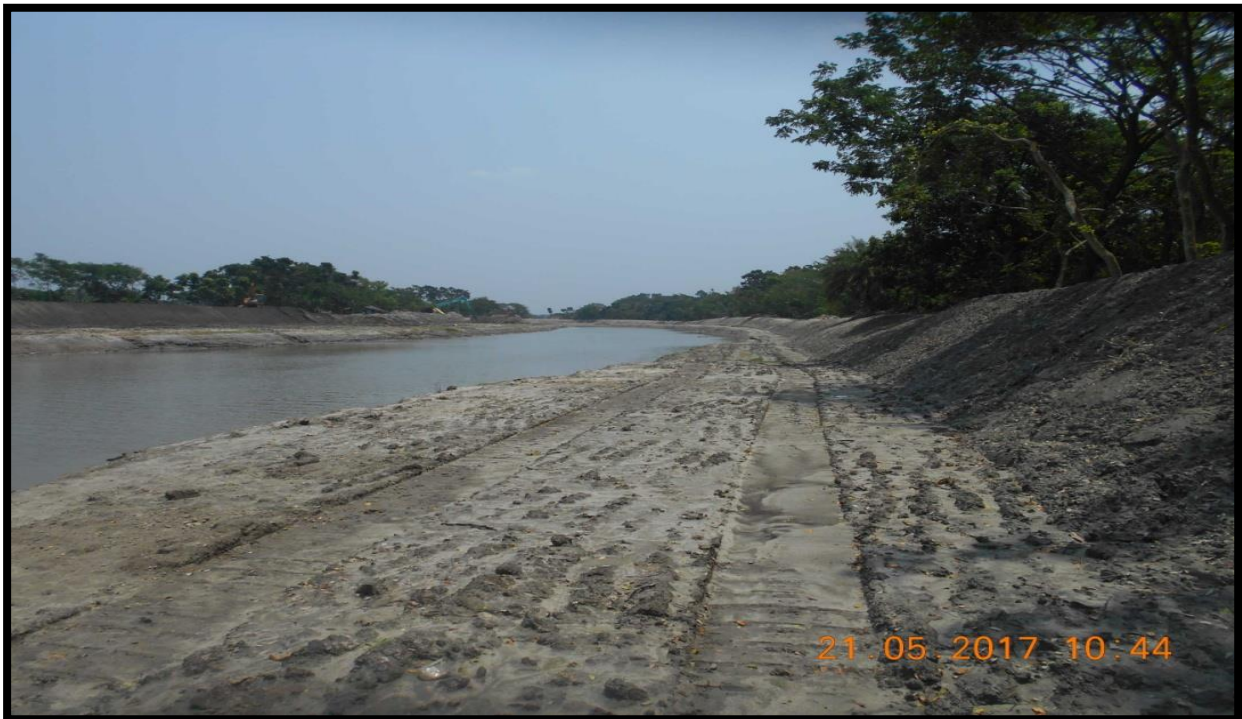
RIGHT BANK AT CHAINAGE 47.5
