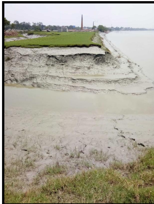
RIVER BANK BREAK AT CHAINAGE 4.5, LEFT BANK
