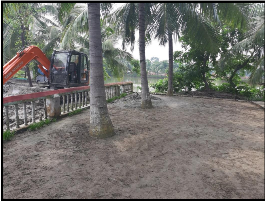
Land acquired by M/s River Waterlink Pvt. Ltd. for RO-RO operations (Pic-3)
