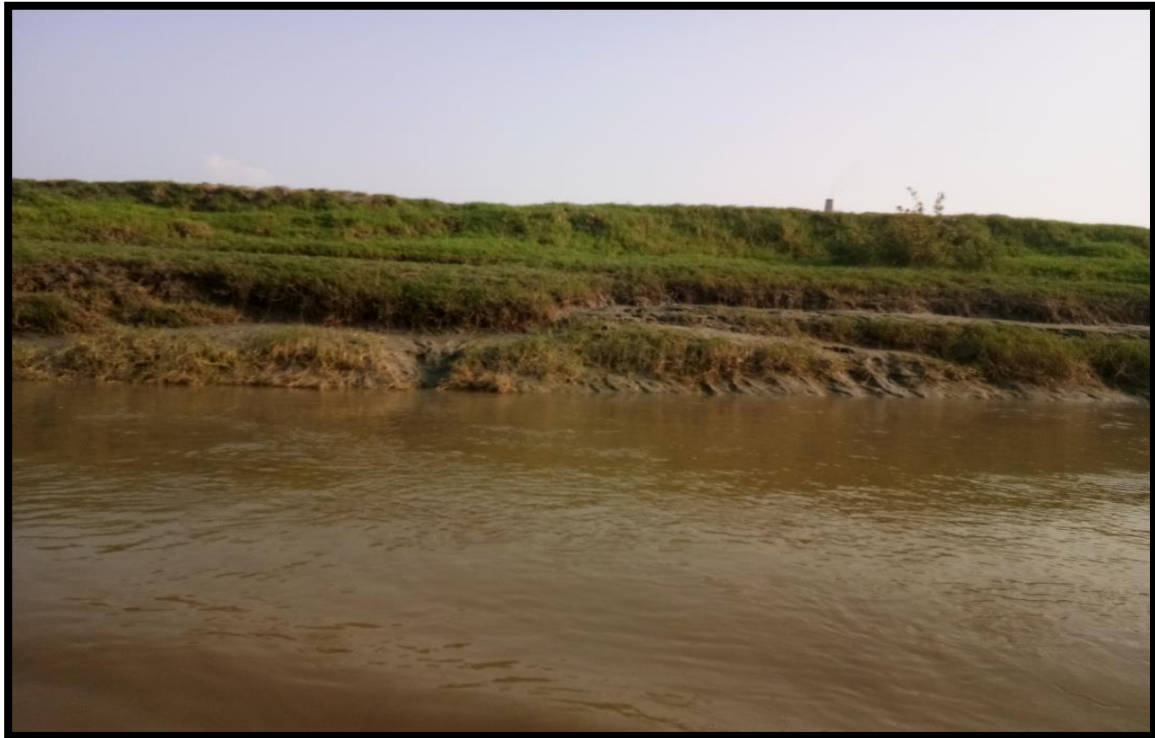
RIGHT BANK AT CHAINAGE 15.9
