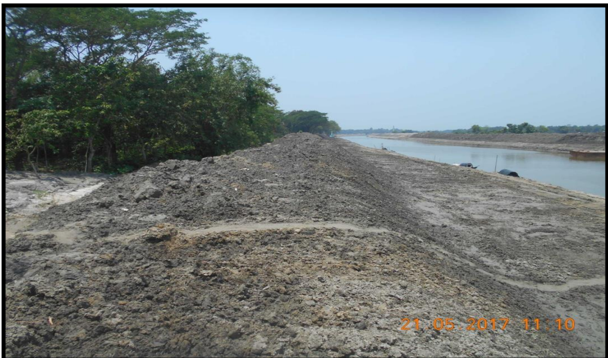
RIGHT BANK AT CHAINAGE 47.7
