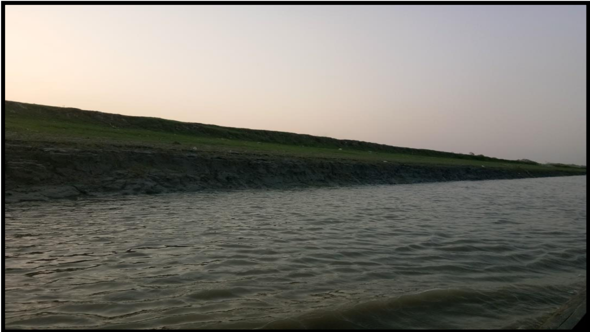
RIGHT BANK AT CHAINAGE 19.7
