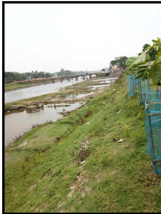
RIGHT BANK AT CHAINAGE 62
