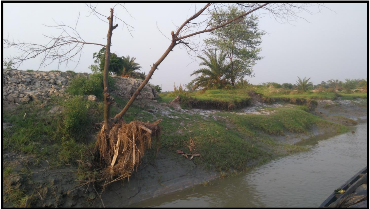
RIGHT BANK AT CHAINAGE 35
