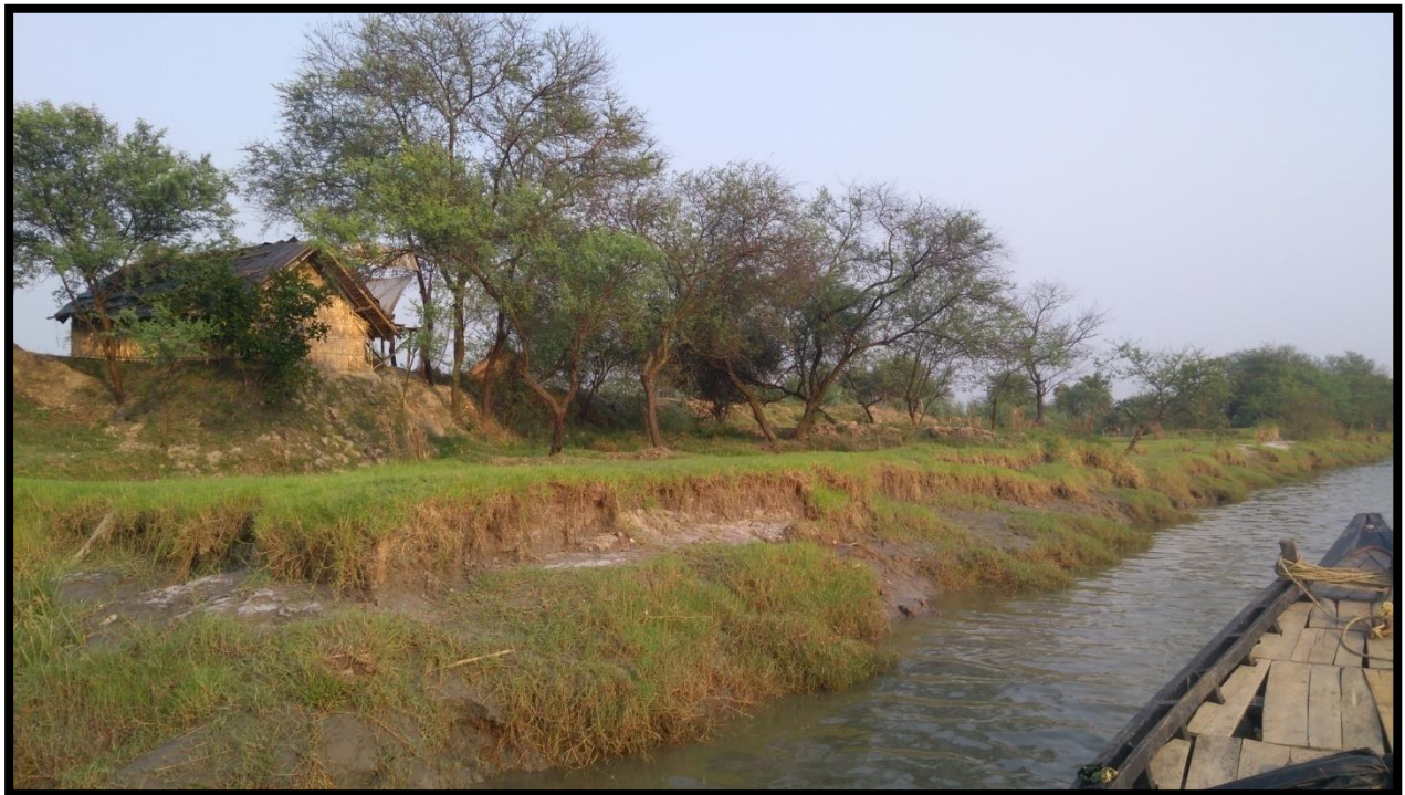
RIGHT BANK AT CHAINAGE 36.5
