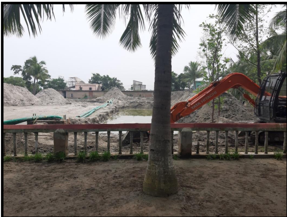
Land acquired by M/s River Waterlink Pvt. Ltd. for RO-RO operations (Pic-2)
