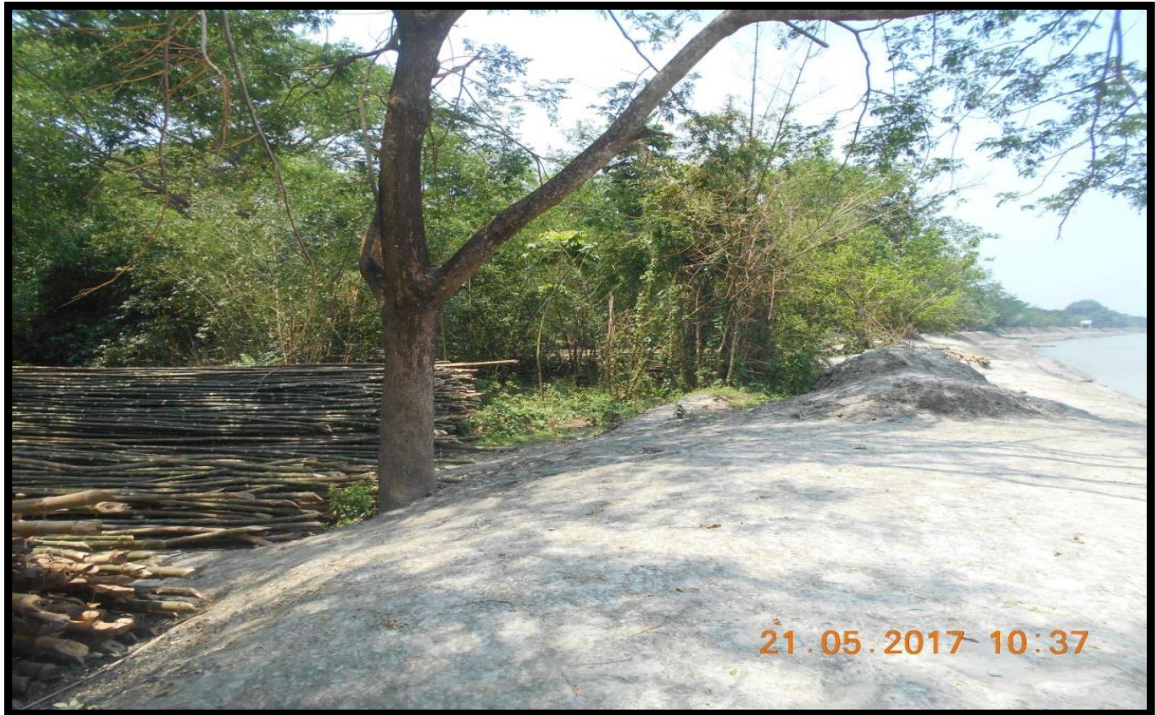
RIGHT BANK AT CHAINAGE 48
