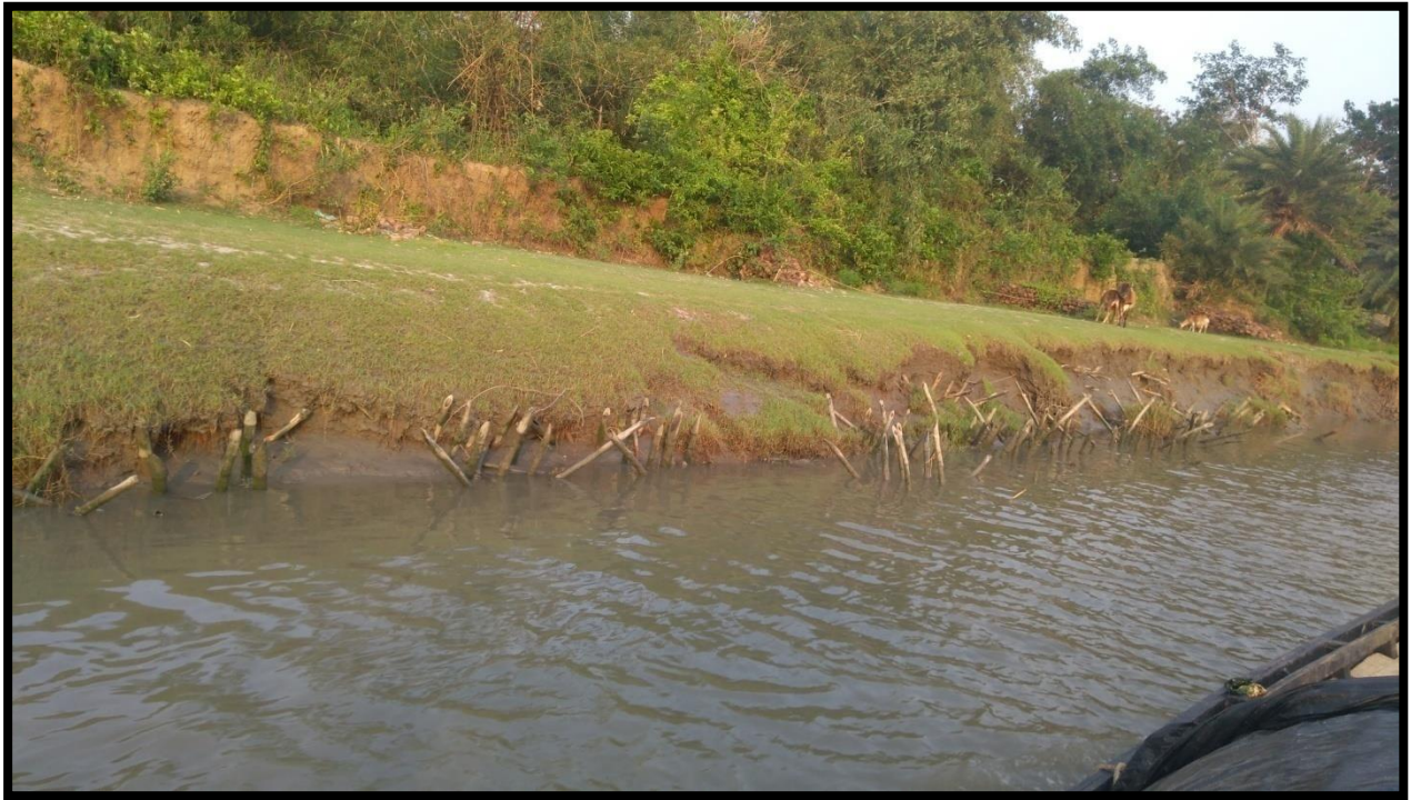
RIGHT BANK AT CHAINAGE 33.5
