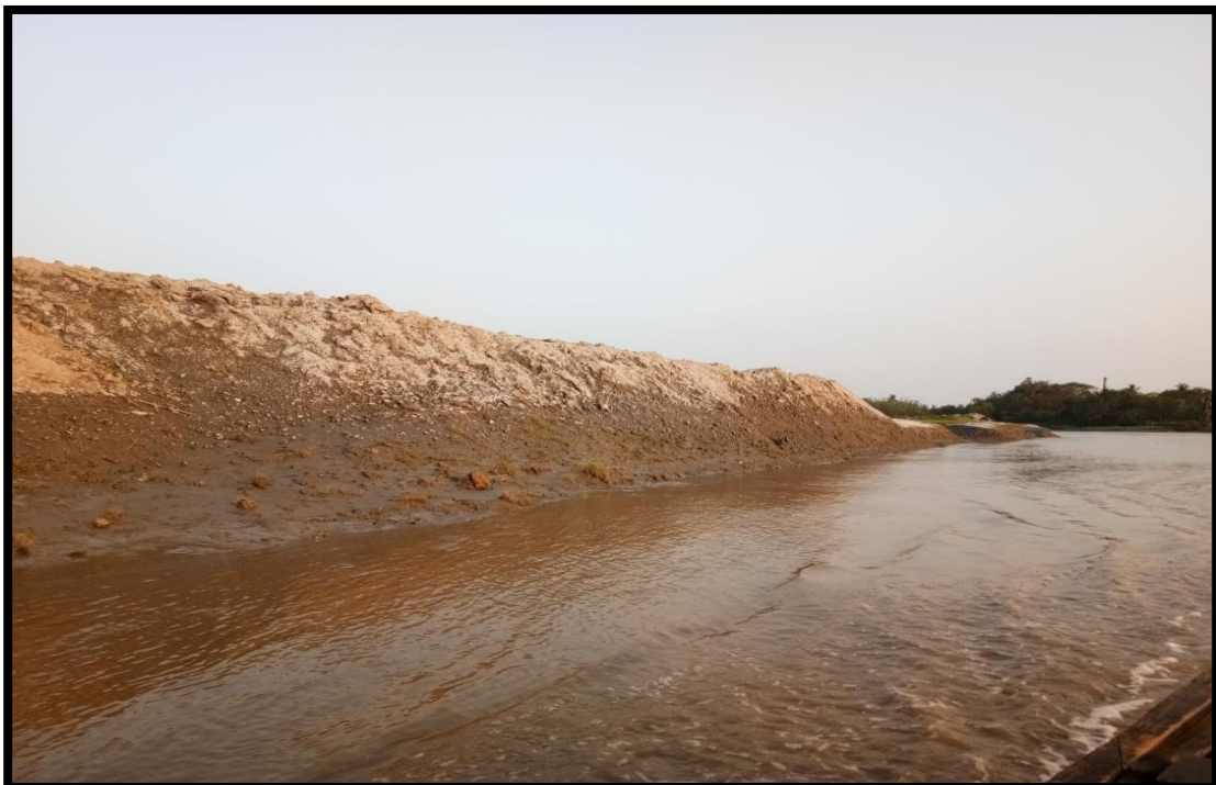
RIGHT BANK AT CHAINAGE 19.3
