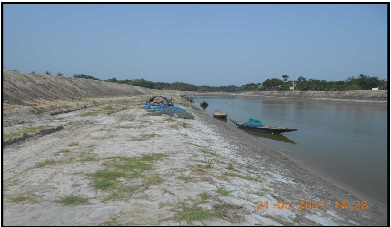
RIGHT BANK AT CHAINAGE 49.1
