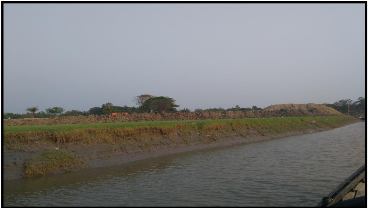
RIGHT BANK AT CHAINAGE 35.5
