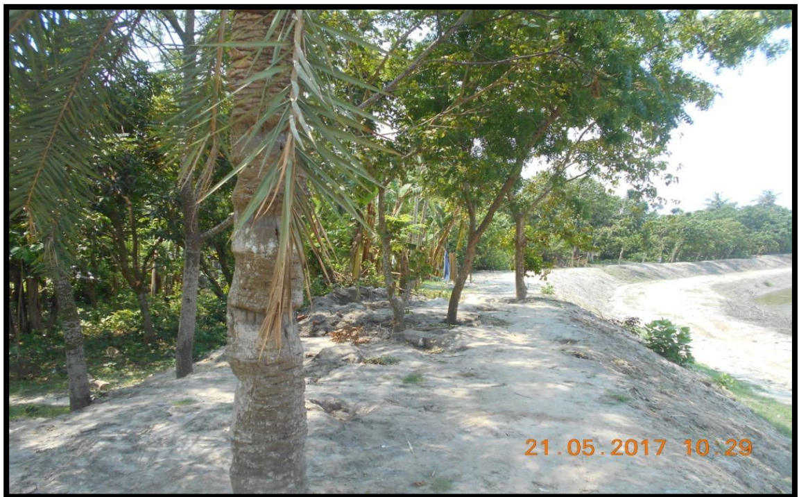
RIGHT BANK AT CHAINAGE 48.5
