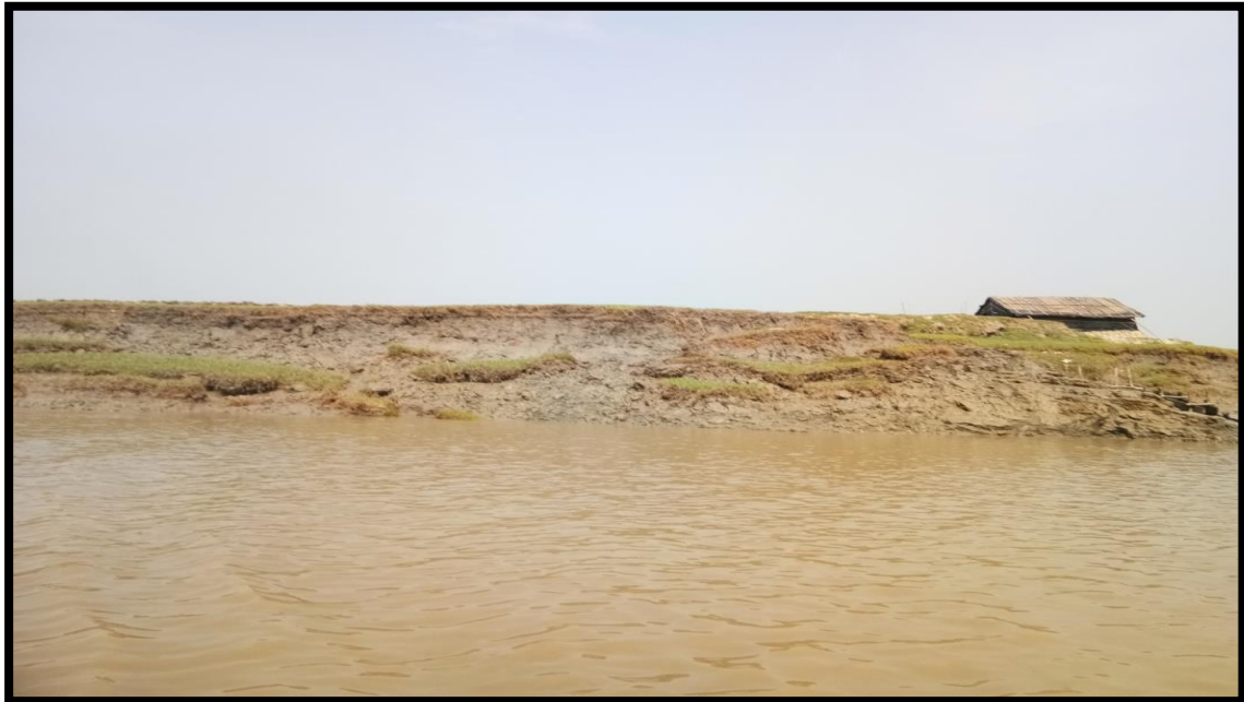
RIGHT BANK AT CHAINAGE 10.5
