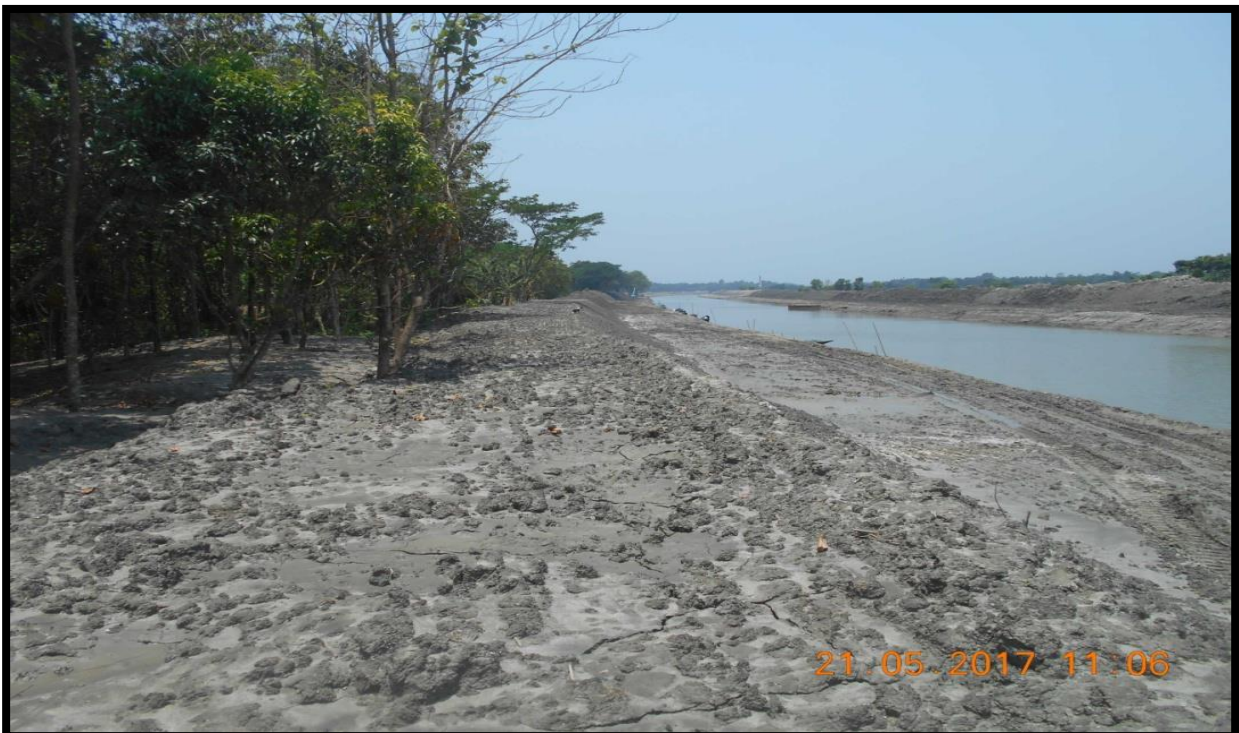
RIGHT BANK AT CHAINAGE 47
