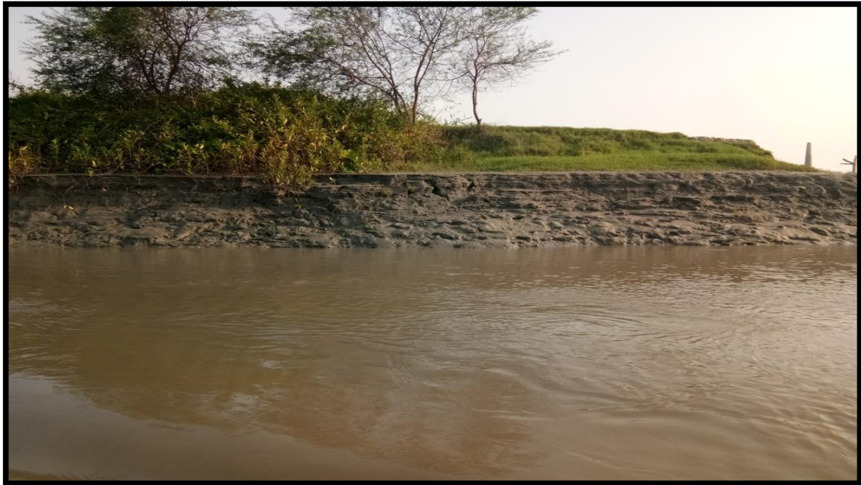
RIGHT BANK AT CHAINAGE 16.5
