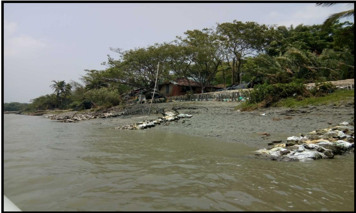
RIGHT BANK AT CHAINAGE 20.5
