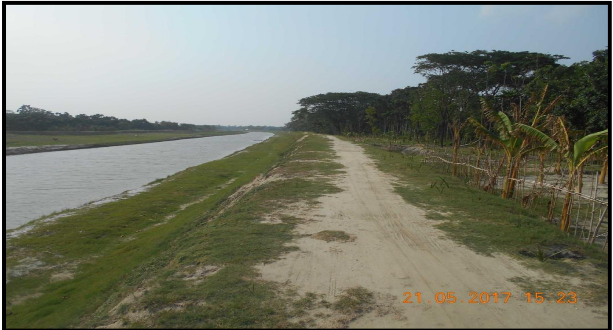
RIGHT BANK AT CHAINAGE 50
