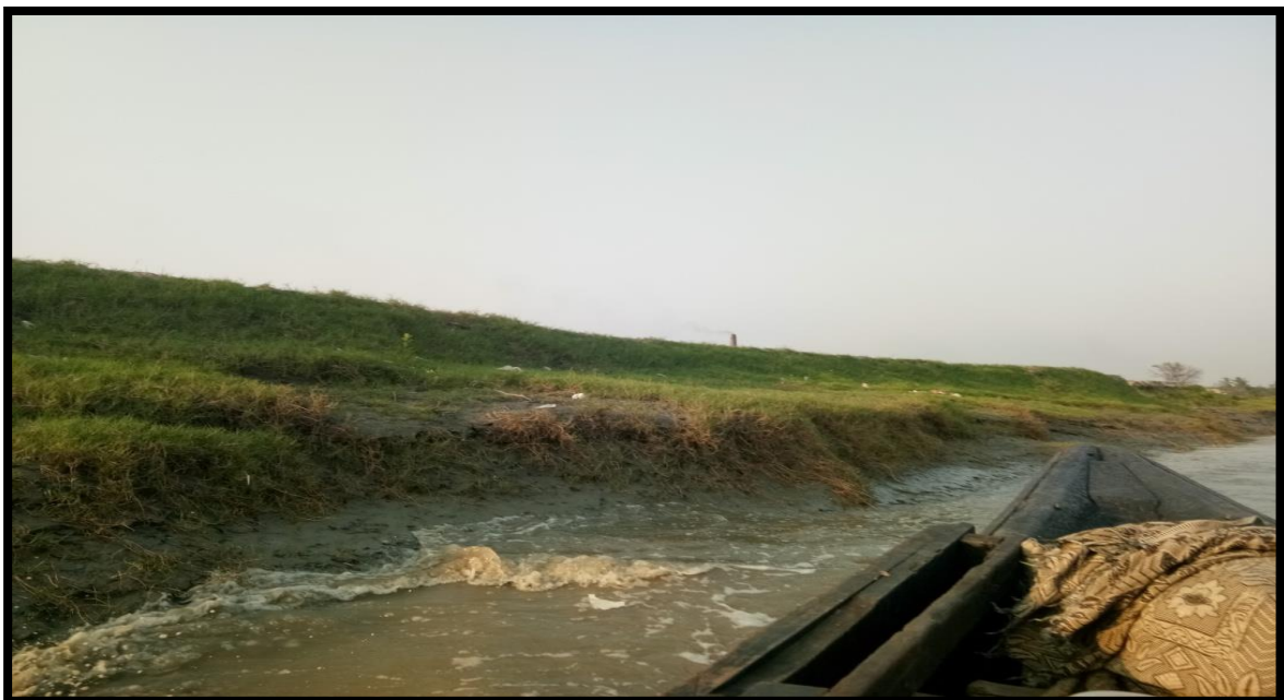
RIGHT BANK AT CHAINAGE 18.1
