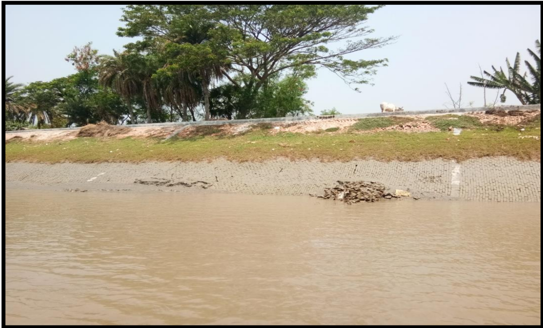
RIGHT BANK AT CHAINAGE 12.5
