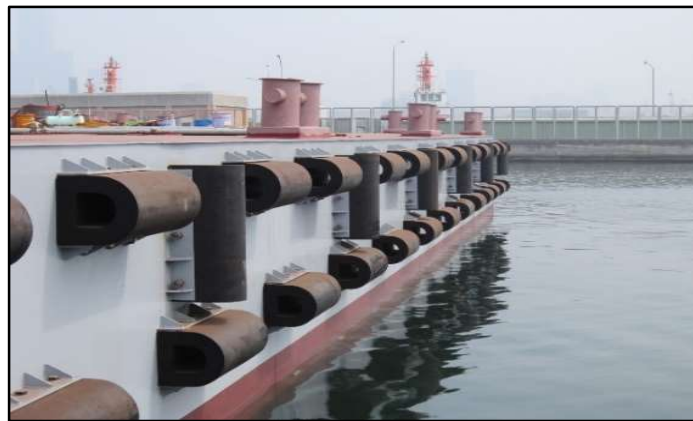
Figure 5.7: D-Type fenders fixed to a quay
