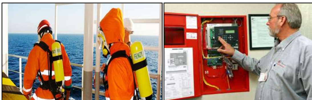
Figure 5.12: EEBD and fire fighters’ outfits & general emergency fire alarm system
