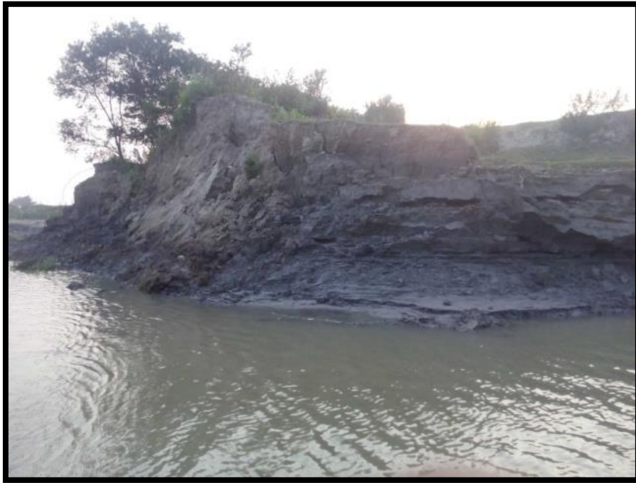
Soil Erosion Area At Chainage 14.0
