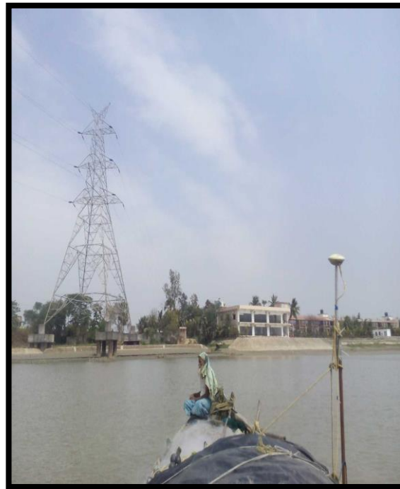
High Transmission Tower at Chainage 34.42
