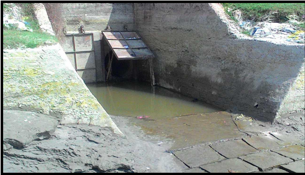
Canal Outlet Gate at RN-04
