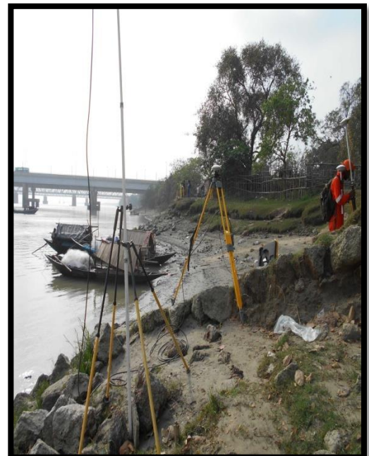
Base Station RN 5-Kolaghat
