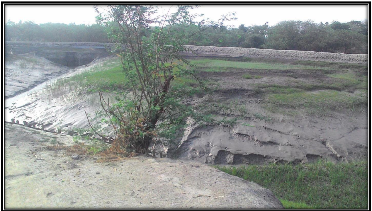
River Bank Erosion near 27.2 CHAINAGE of Left Side of River Bank
