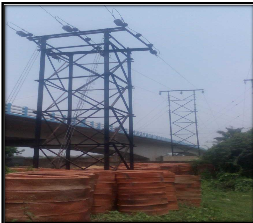
High Tension at CHAINAGE 4.1
