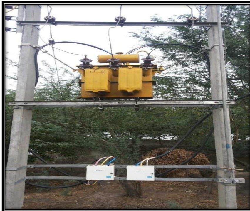
Transformer near 22.5 CHAINAGE of Left Side Of River Bank
