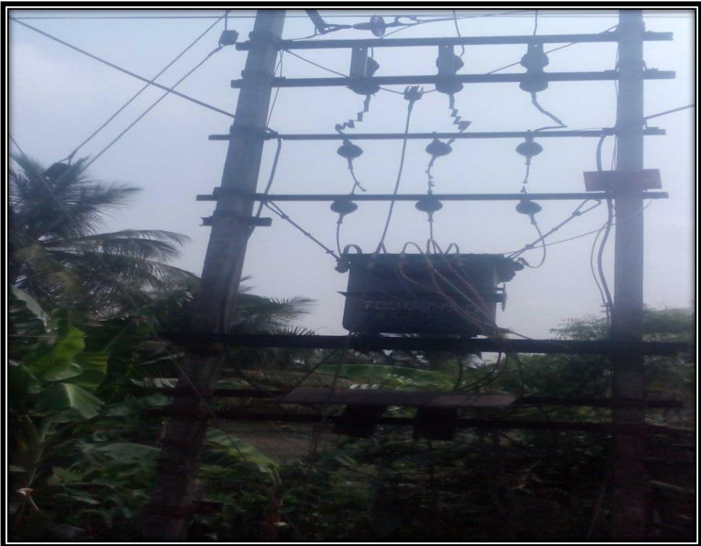
Transformer at CHAINAGE5
