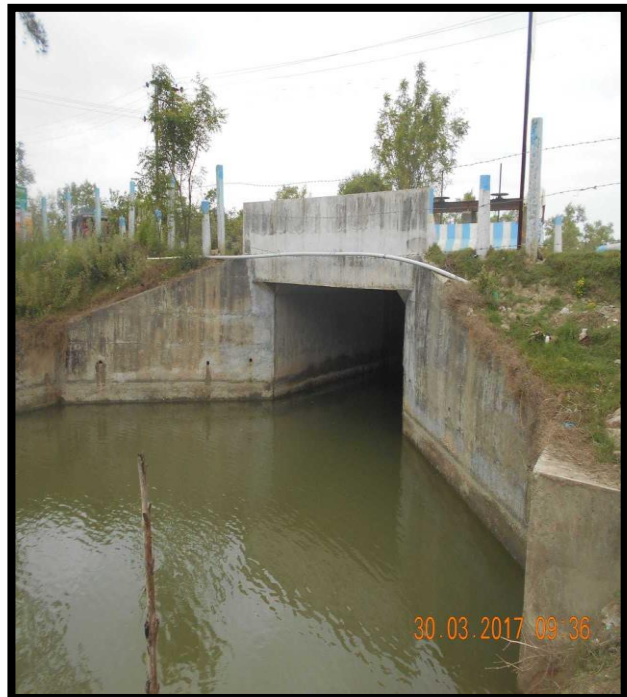
WATER LOCK NEAR ML-01 AT CHAINAGE 58, RIGHT BANK
