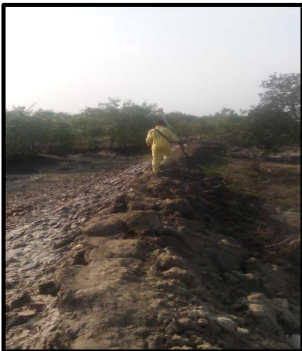
DAMAGED RIVER BANK AT CHAINAGE 65.9, RIGHT BANK
