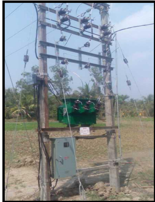
Transformer at Mousani island Chainage 7.5
