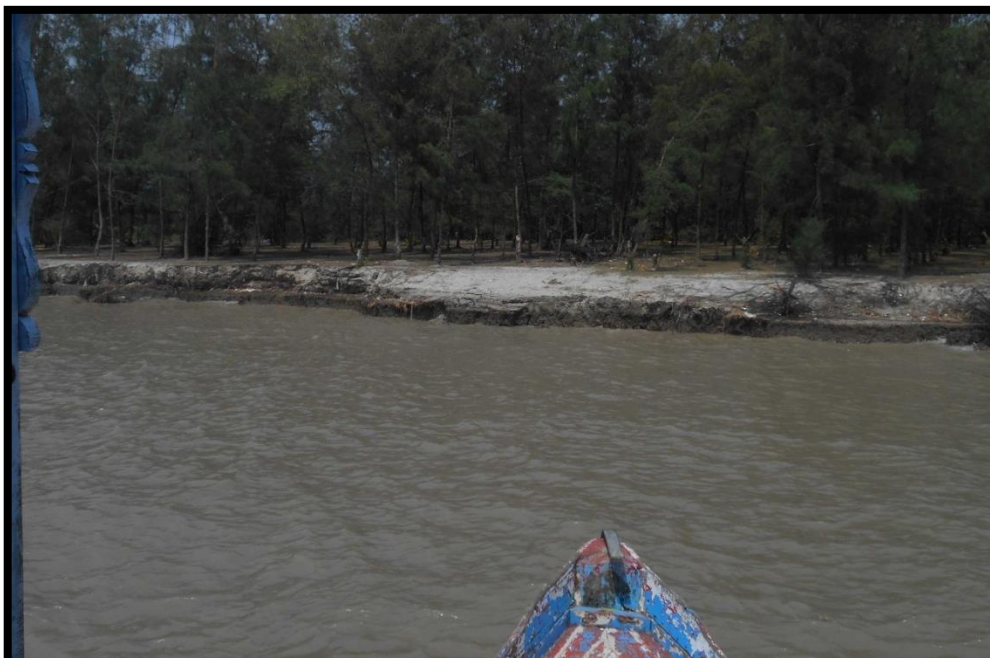
Un Protected Bank at Chainage 22.8
