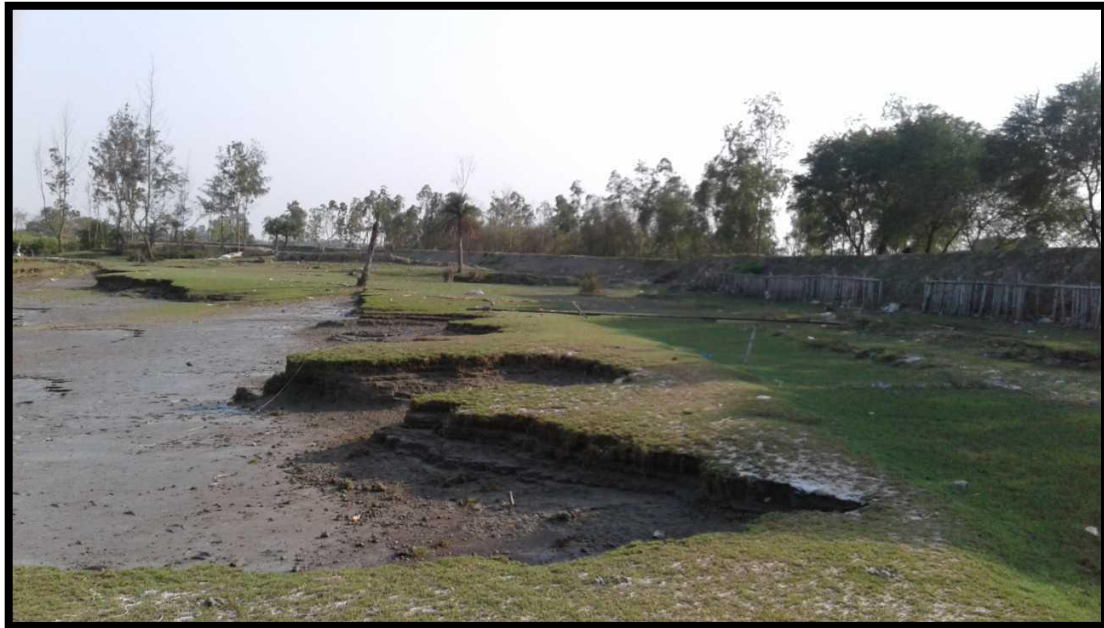
Un Protected Bank at Chainage 23
